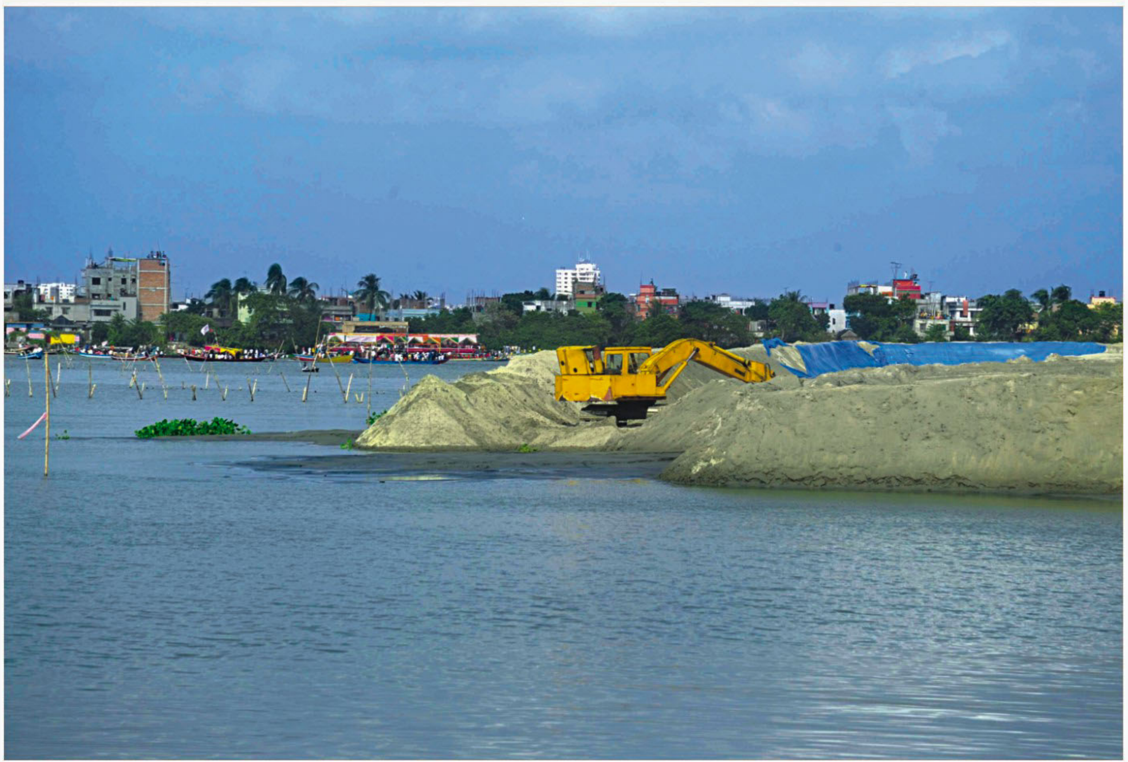
Two private companies are filling up this portion of the Buriganga river at Waaspur on the outskirts of the capital to set up two power plants and an amusement park. A digger is in operation at the site. The bamboo poles sticking out of the water are markers up to which the river would be filled.
