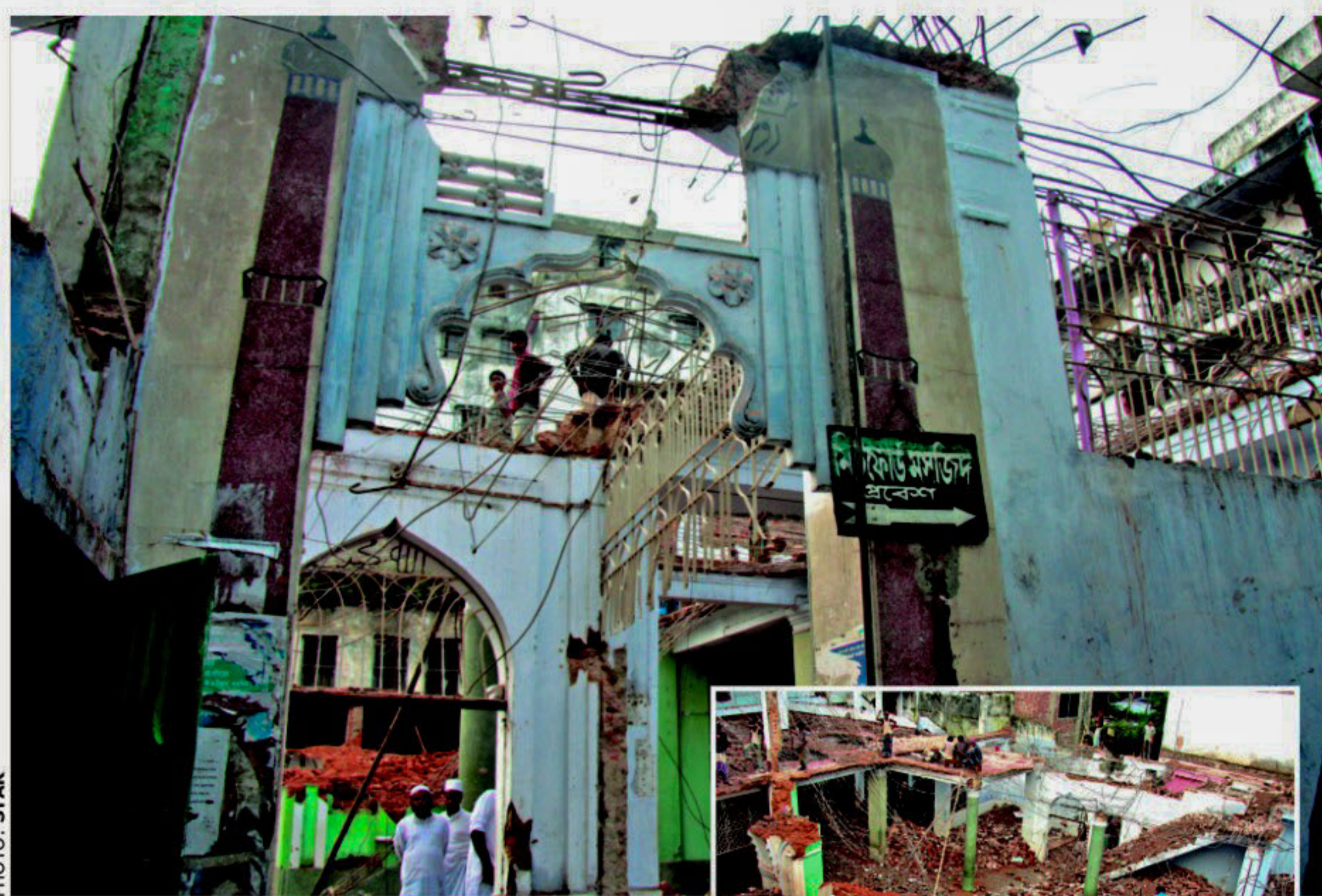
This mosque built in the Mughal period near Mitford Hospital in Old Dhaka is being torn down to make way for a modern one. Inset, workers knocking down structures.
