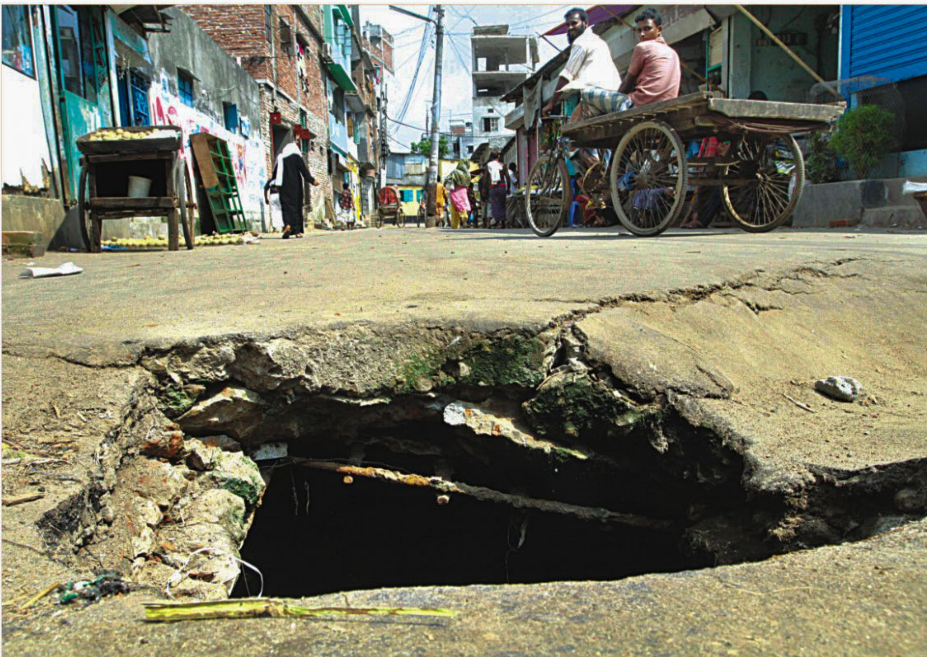
A potential death trap lies in wait for the unsuspecting pedestrian, especially after dark, as the lid of this manhole in Paschim Shahidnagar area in the city's Lalbagh went missing a long time ago. The photo was taken yesterday.
