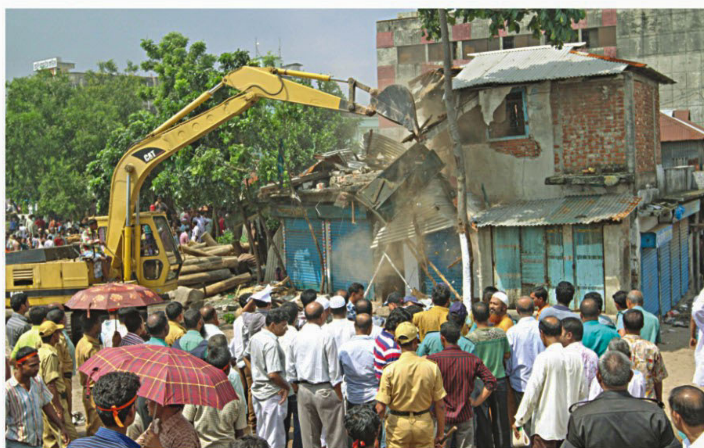
PHOTO: PHOTO An excavator demolishes illegal structures on Beribadh area, East of Shyambazar and adjacent to the river Buriganga, during an eviction drive by Dhaka District Administration, Bangladesh Inland Water Transport Authority and Roads and Highways Department yesterday.
