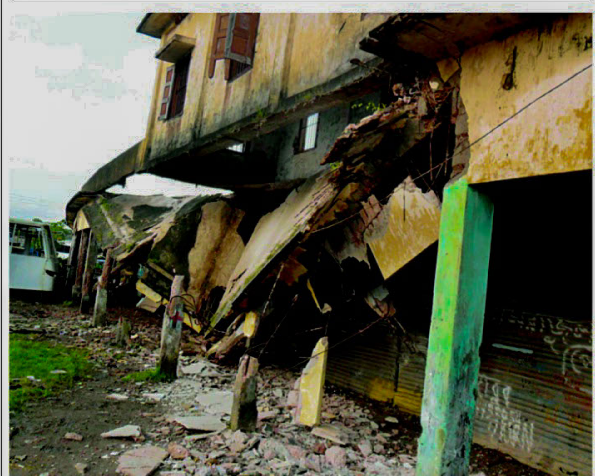
Left without any repair for long, Patuakhali district stadium partially collapsed on Saturday. Built in 1978, the 35,000 square feet stadium hardly saw any renovation allegedly due to lack of fund.
