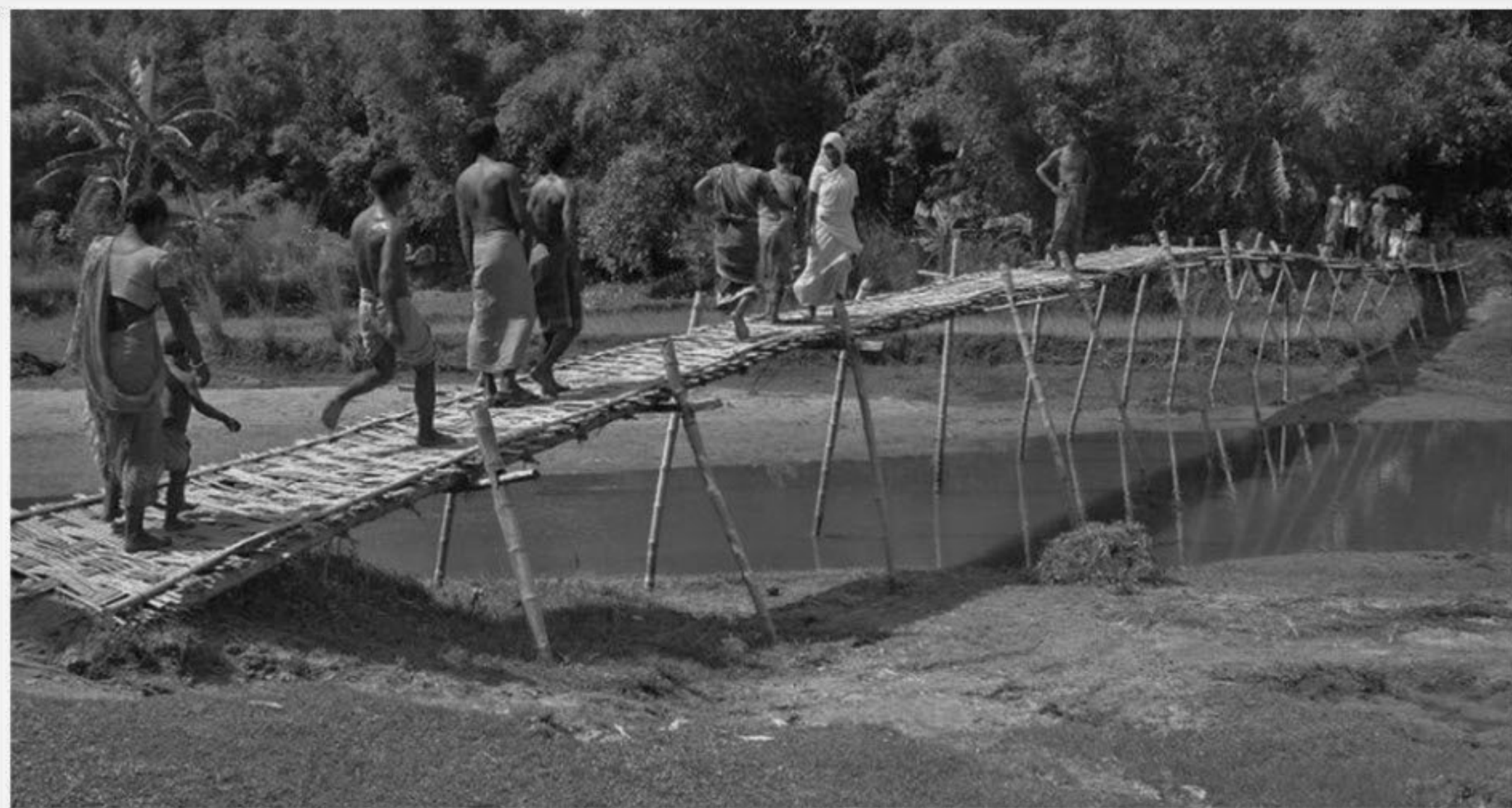
Built by local women, this bamboo bridge over Chekadara River flowing between Nayani Bagdogra and Bagdogra villages in Domar upazila in Nilphamari district serves thousands of people of several villages, especially schoolchildren, on both sides of the river.
