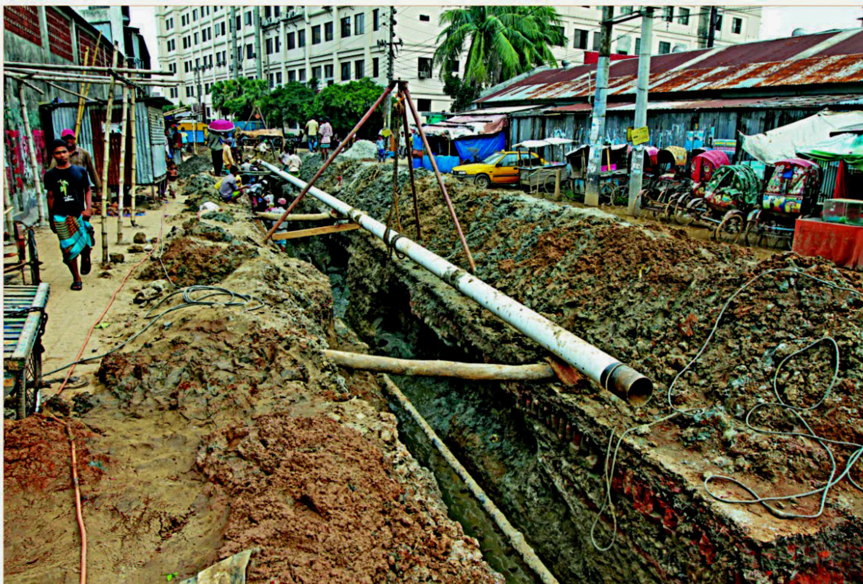
This road on Begunbari in Tejgaon Industrial Area in the city made completely unusable as Titas Gas Transmission and Distribution Company Limited dug it up to install pipes to supply gas, causing suffering to the locals.
