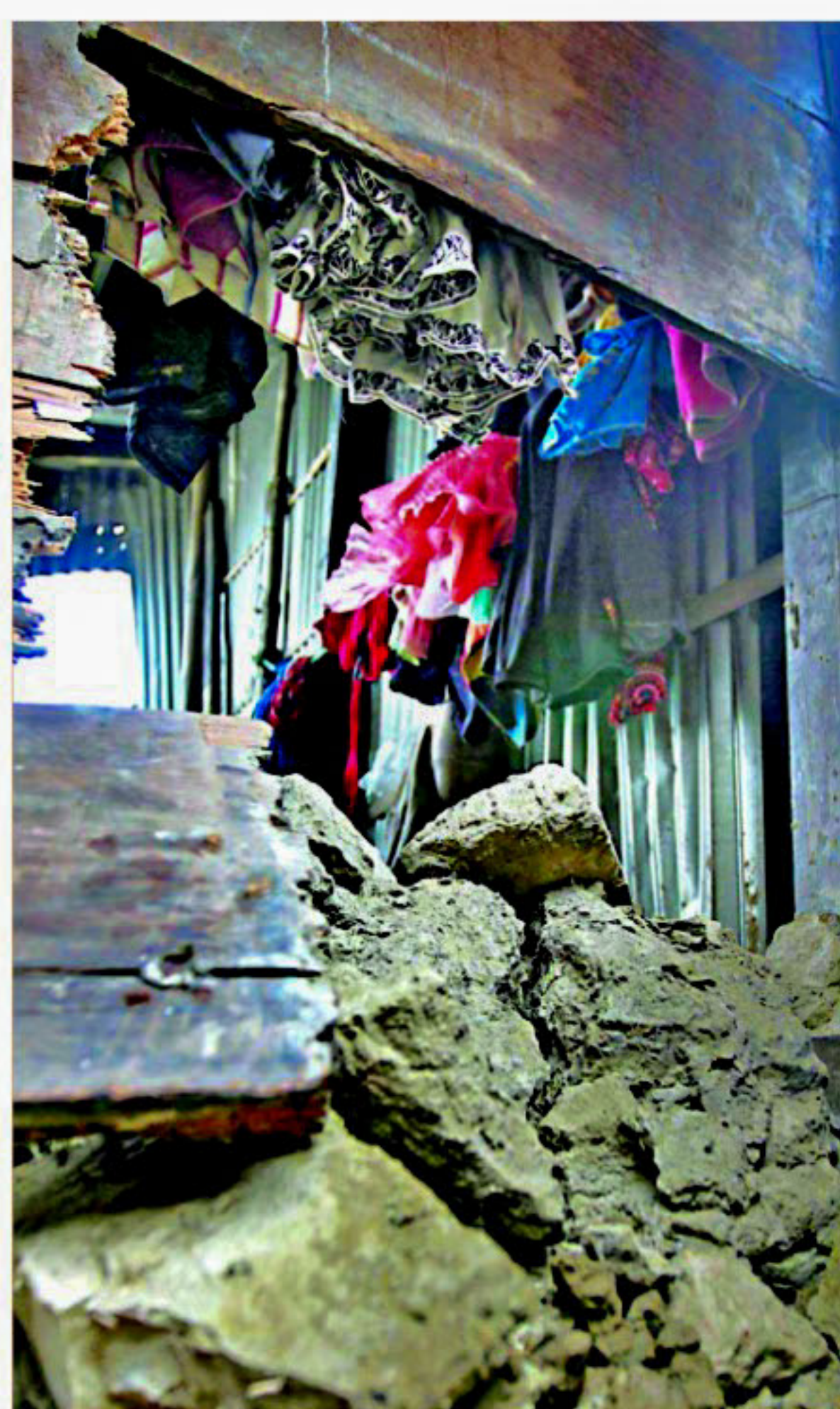
PHOTO: ANURUP KANTI DAS Wall of a mud house collapses at Dwipkalar Morol village under Patiya upazila in Chittagong early yesterday, leaving three of a family killed and two others injured.
