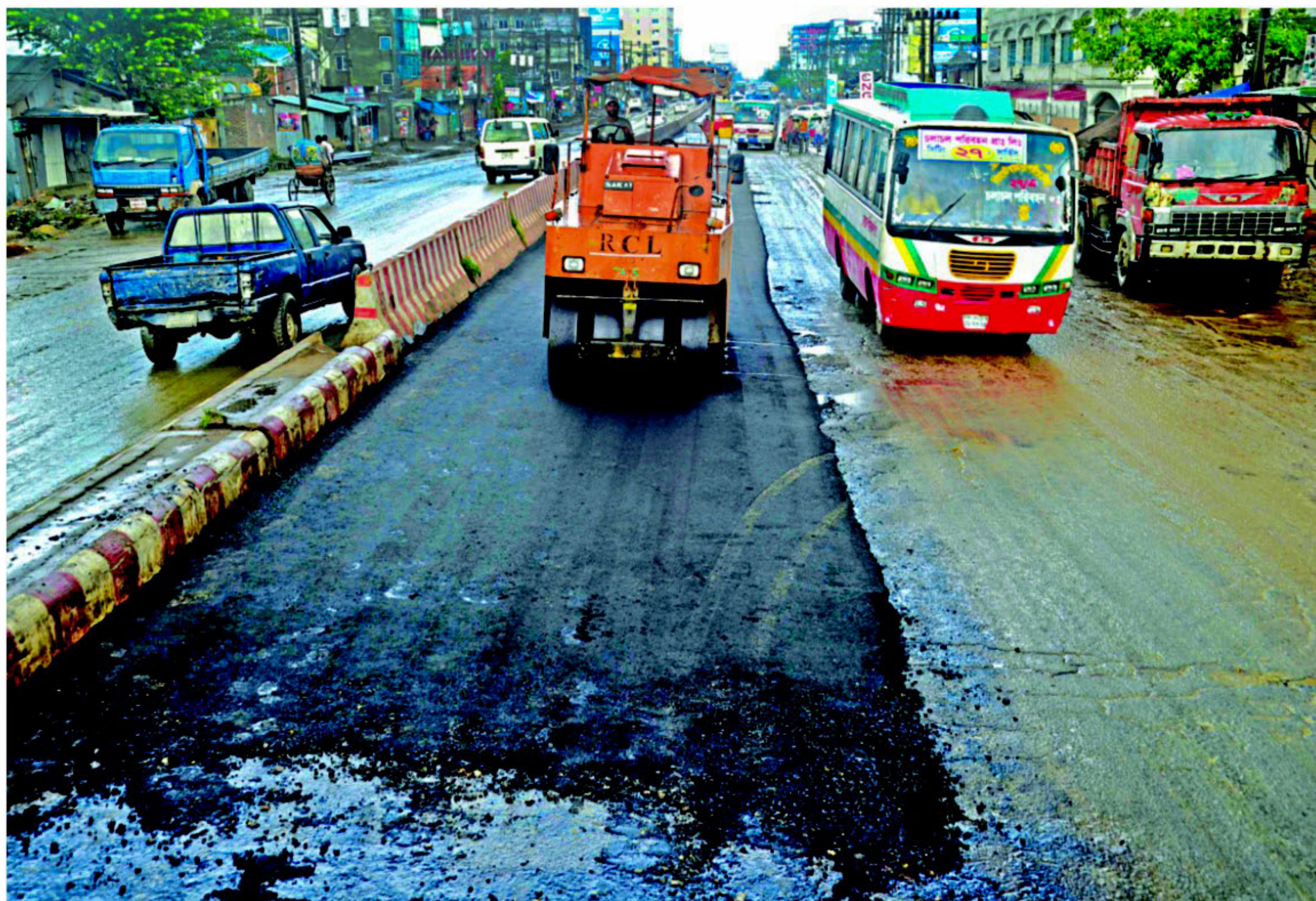
Renovation of Dhaka-Mymensingh highway continues at Sign Board in Gazipur yesterday. Transport owners last month stopped bus operation on the route for several days demanding its overhaul.
