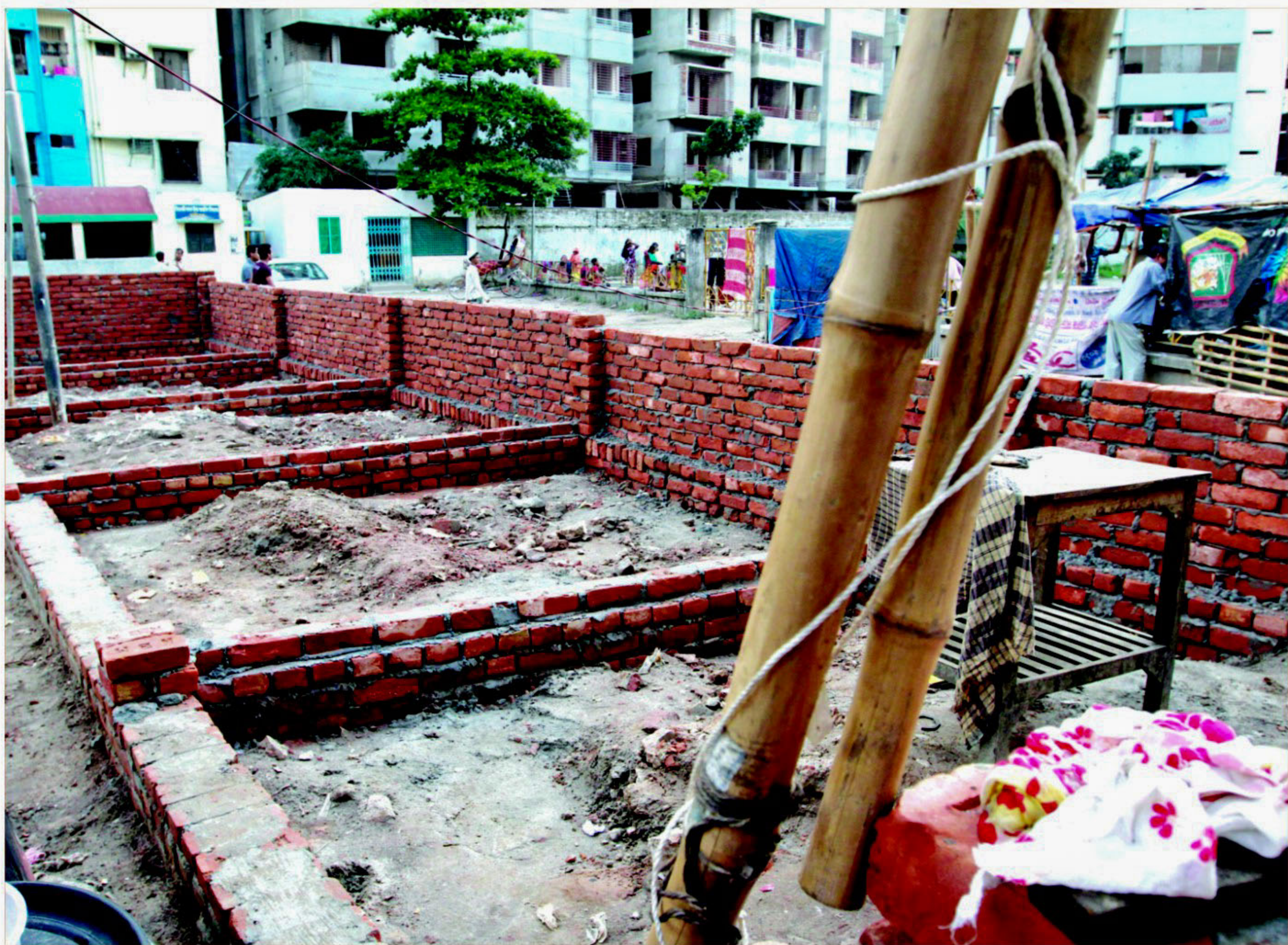
Eight shops being constructed on the playground of Siddheswari Boys' Higher Secondary School in the city after the management committee leased out the space to meet fund shortages. The photo was taken yesterday.
