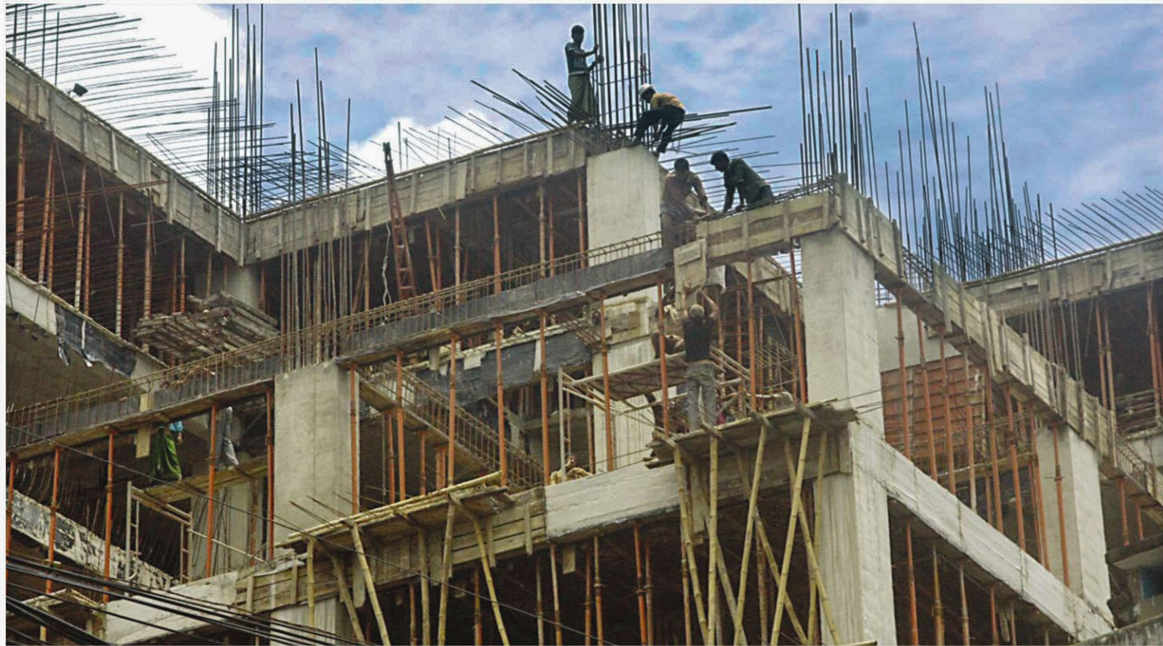
Workers at work without safety measures in a construction site in the port city.
