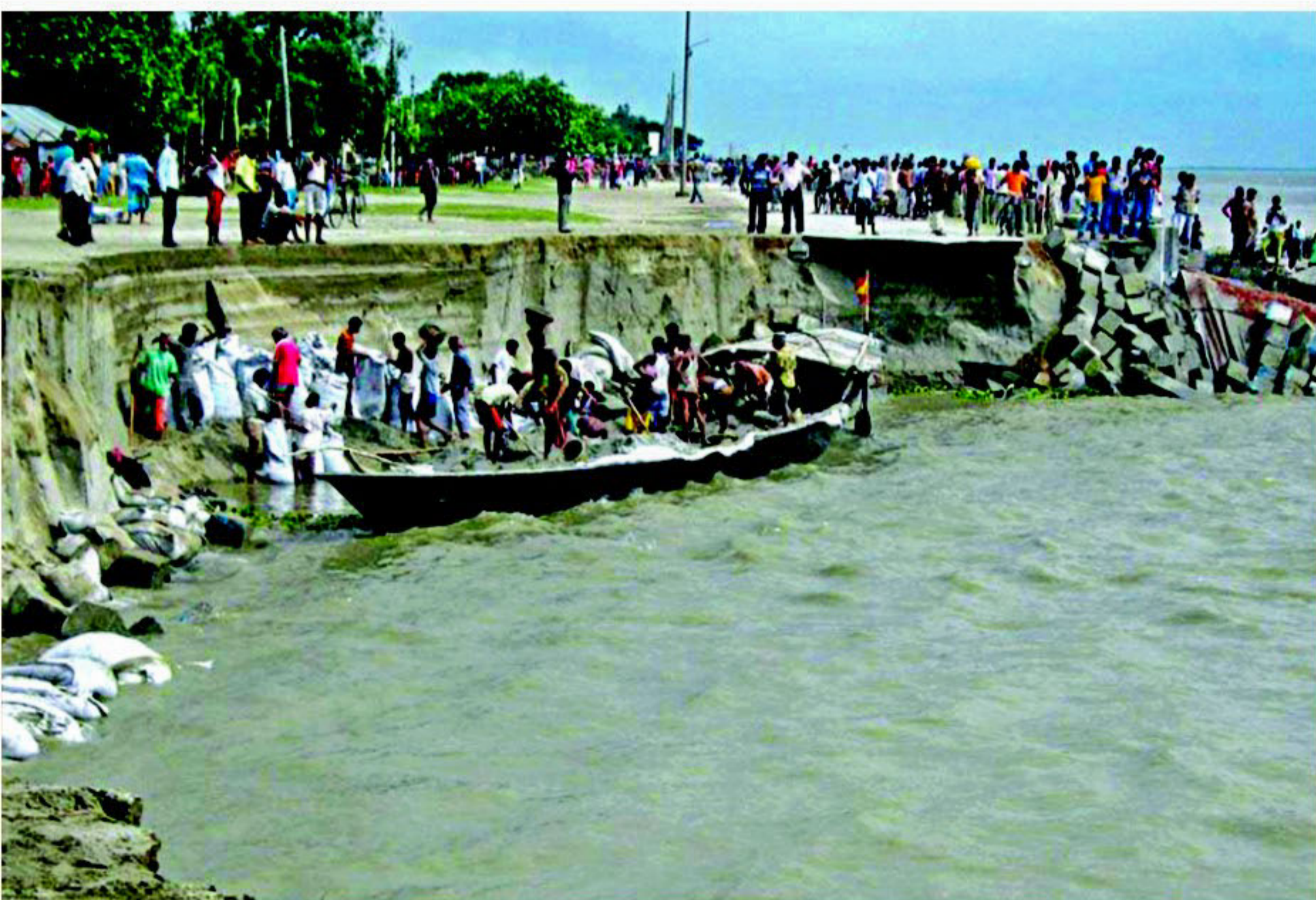
Locals try to stop the Jamuna from eroding the Sirajganj town protection embankment yesterday with sandbags. Four days ago the river damaged another point of the embankment. Story on page 1.
