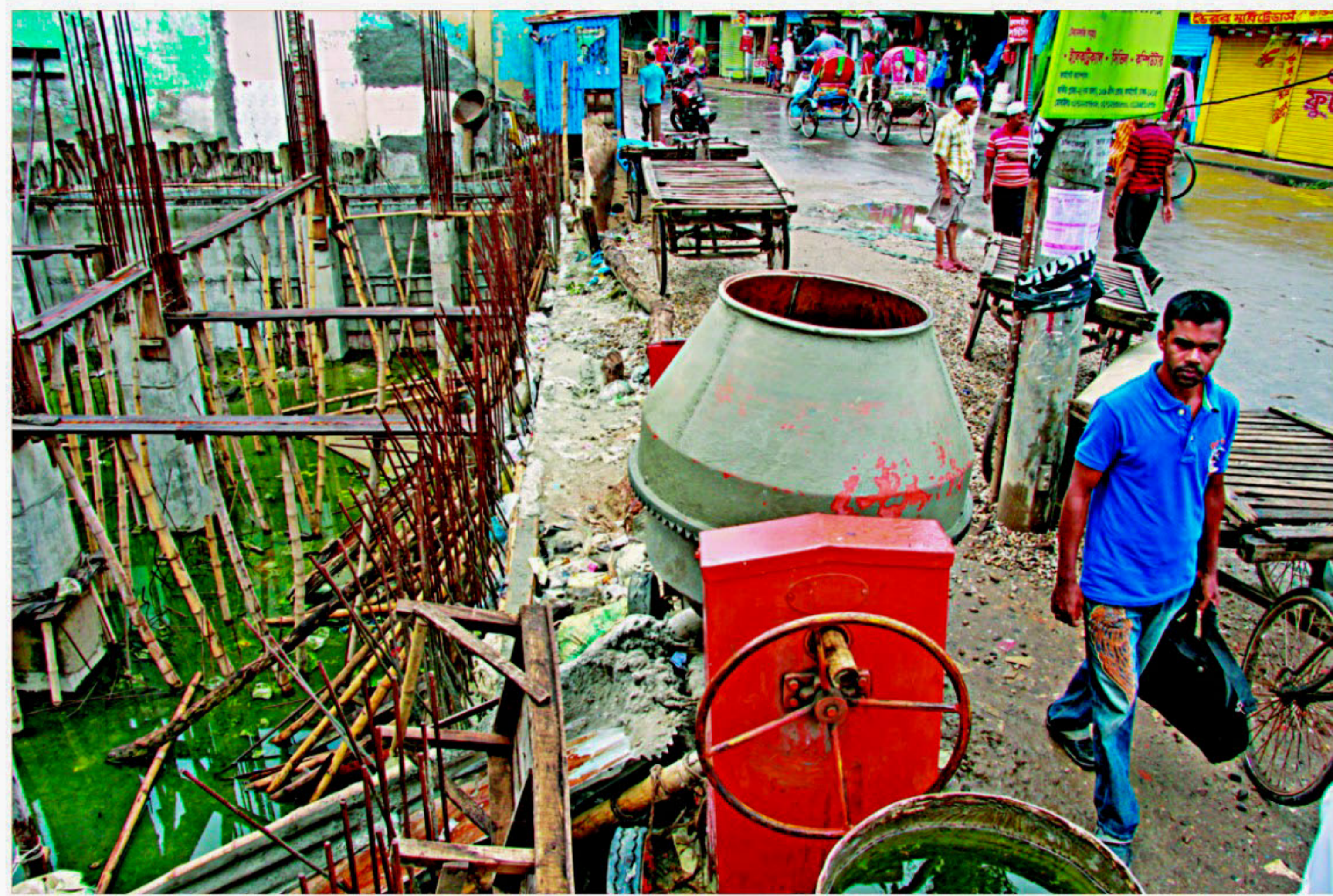
Founding of a multi-storied building in front of Tejturi Bazar Rail Gate in the city's Tejgaon is being done without any safety measures while keeping construction materials on the road blocking the footpath. The photo was taken yesterday.
