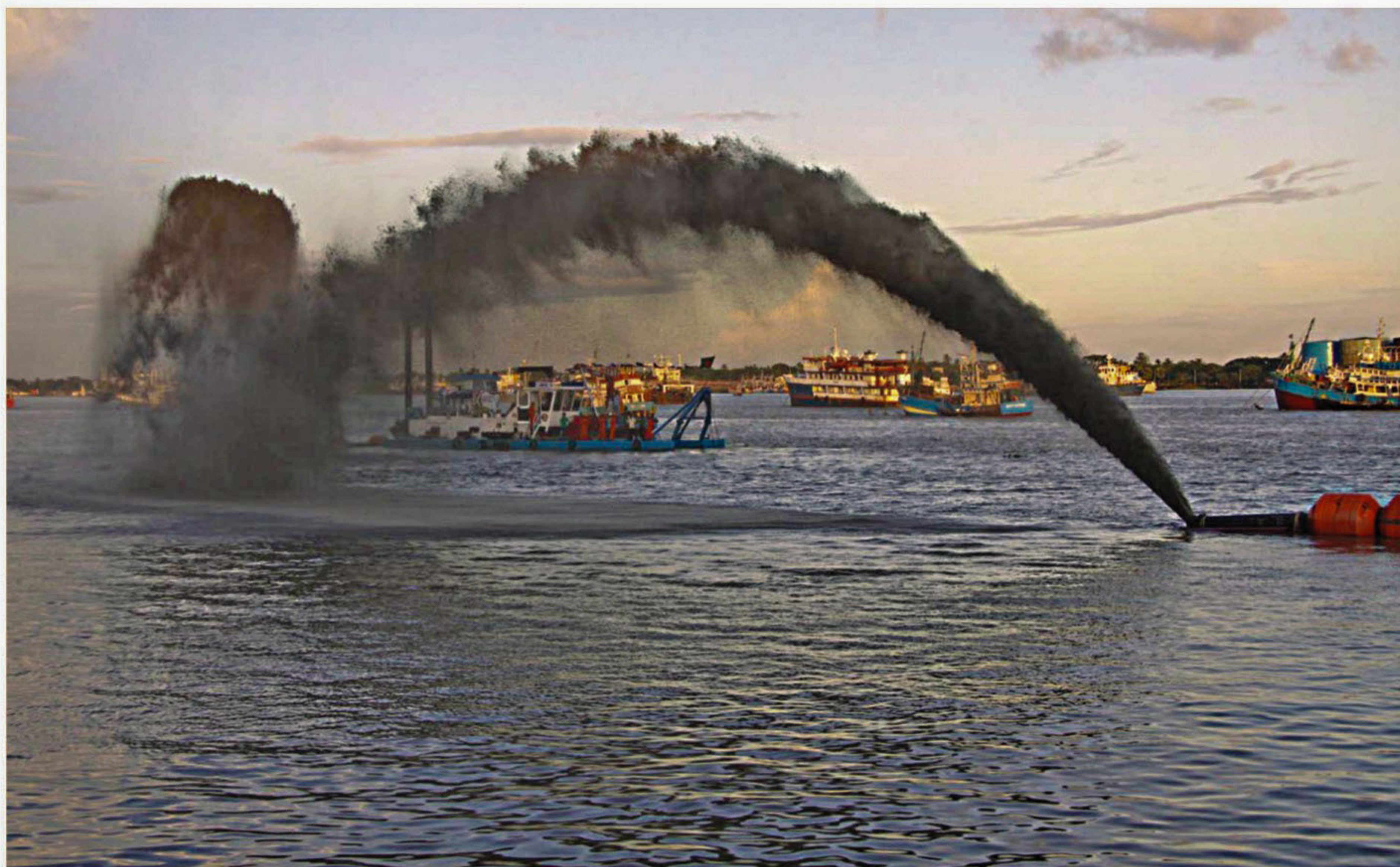
The long-awaited capital dredging in the river Karnaphuli begins after Shipping Minister Shahjahan Khan inaugurated the project in Chittagong yesterday.
