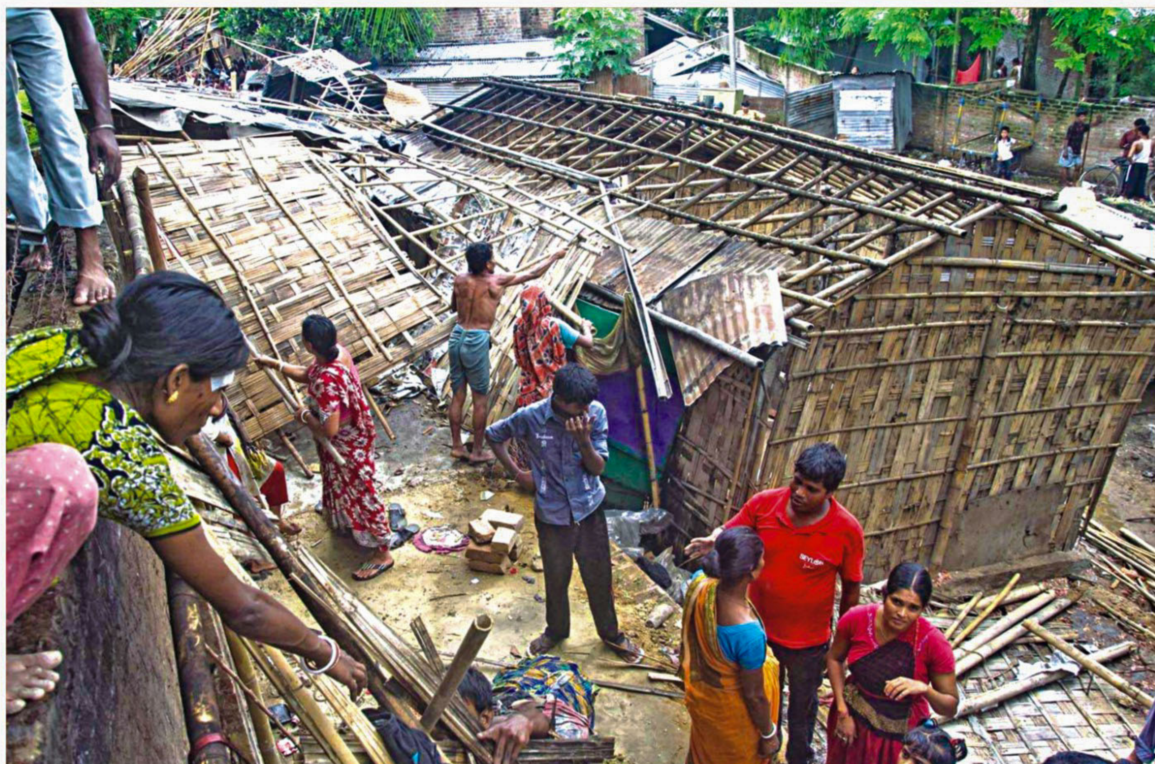
Slum dwellers voluntarily dismantle their makeshift homes at Raiway Hospital Colony in CRB area of Chittagong yesterday when Bangladesh Railway authorities went there on an eviction drive.
