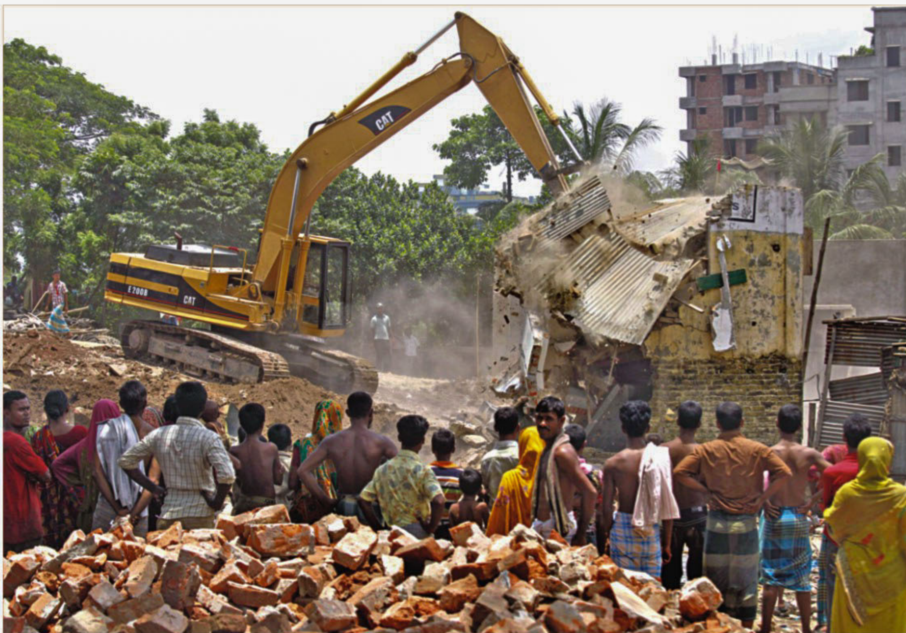
Bangladesh Water Development Board demolishes illegal structures on both sides of Mohammadpur Beribadh road in the city yesterday.
