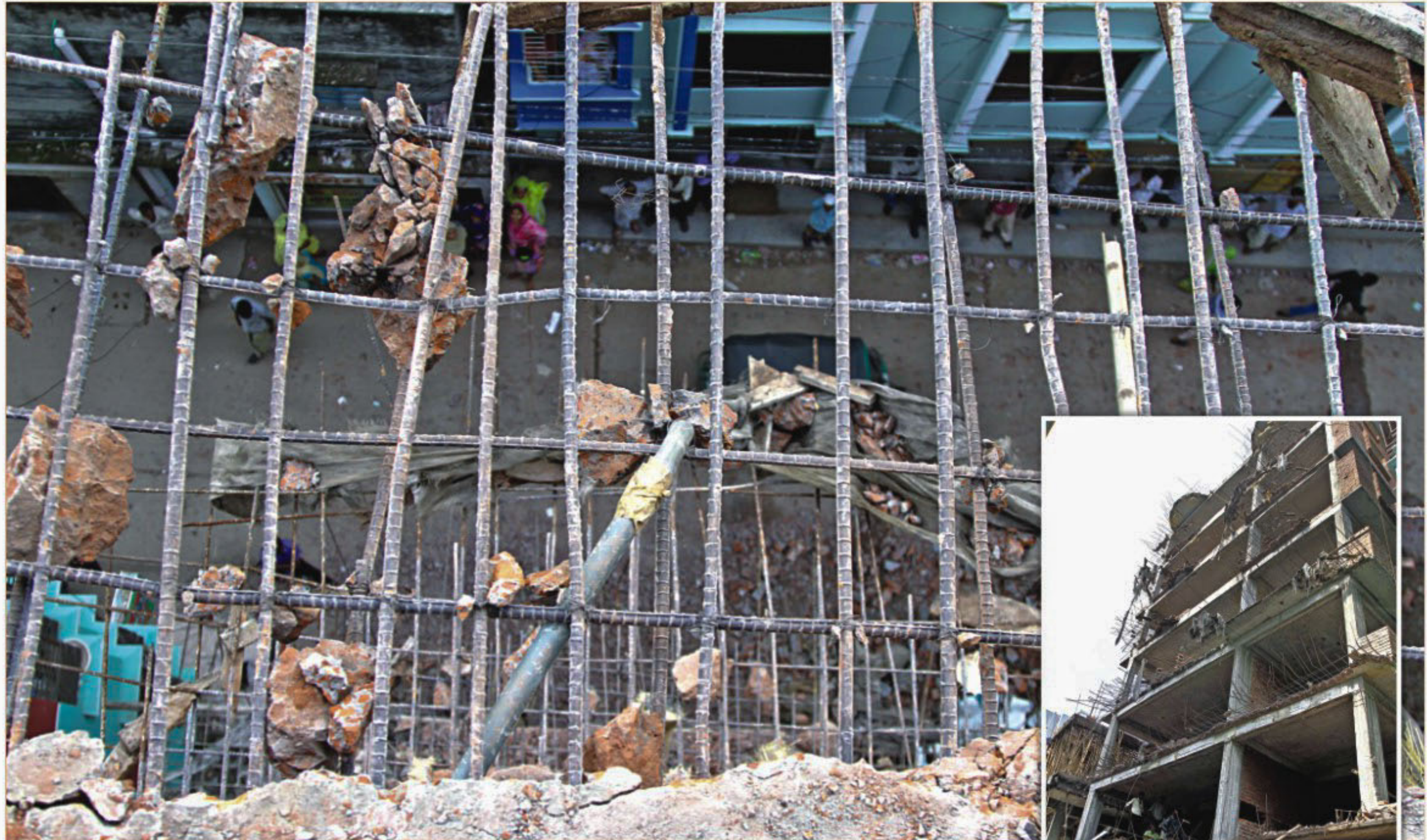
A breath of wind could send these chunks of concrete stuck to the iron rods tumbling down on pedestrians oblivious to the danger from above. A mobile court yesterday demolished the unauthorised extensions of the building in the city's Madhya Badda scattering debris on the street.
