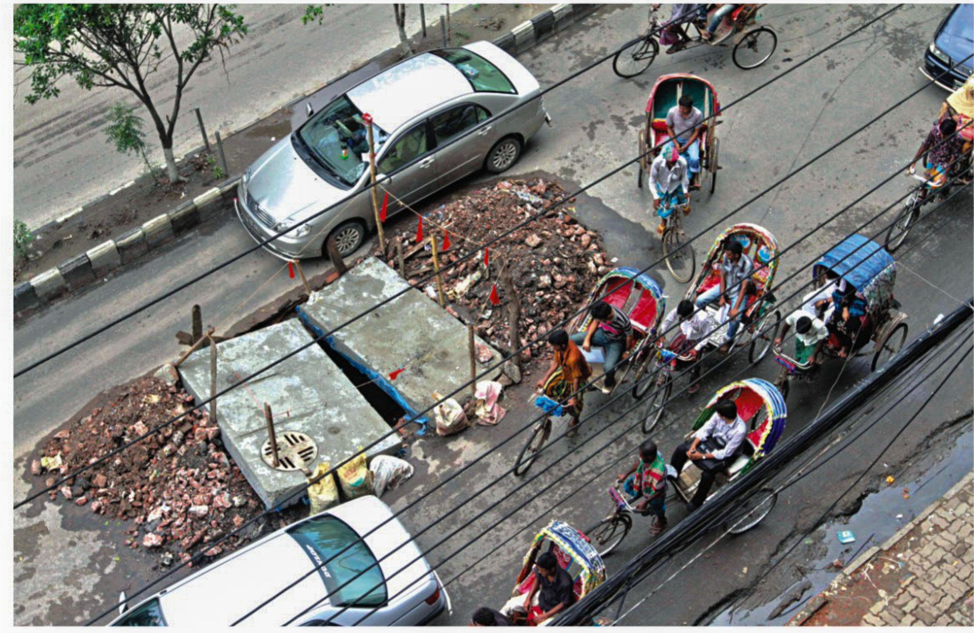
The repair work for concrete lids is obstructing traffic flow on Selina Parveen Road at the capital's Moghbazar. Locals allege the slabs are found broken within a few days of their repair. They wish the authorities speed up the work and do it properly this time.
