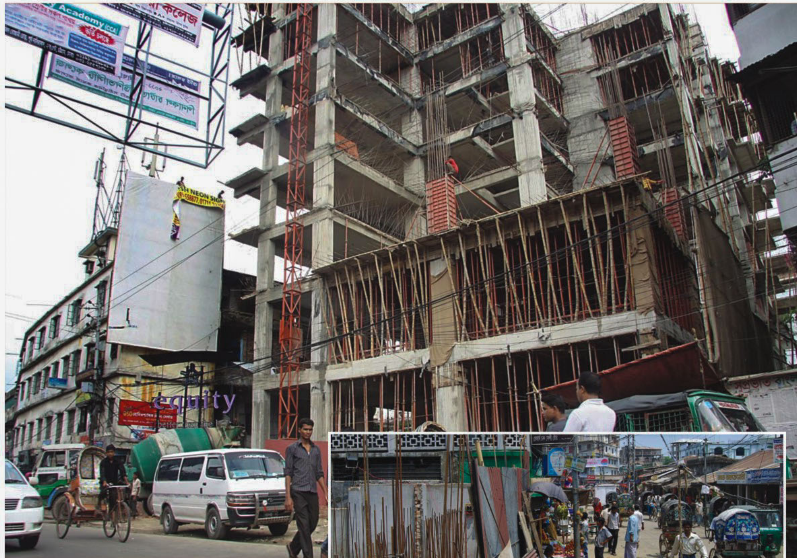
A multi-storey building is being constructed at Momin Road in the port city without any safety measure while the footpath.
