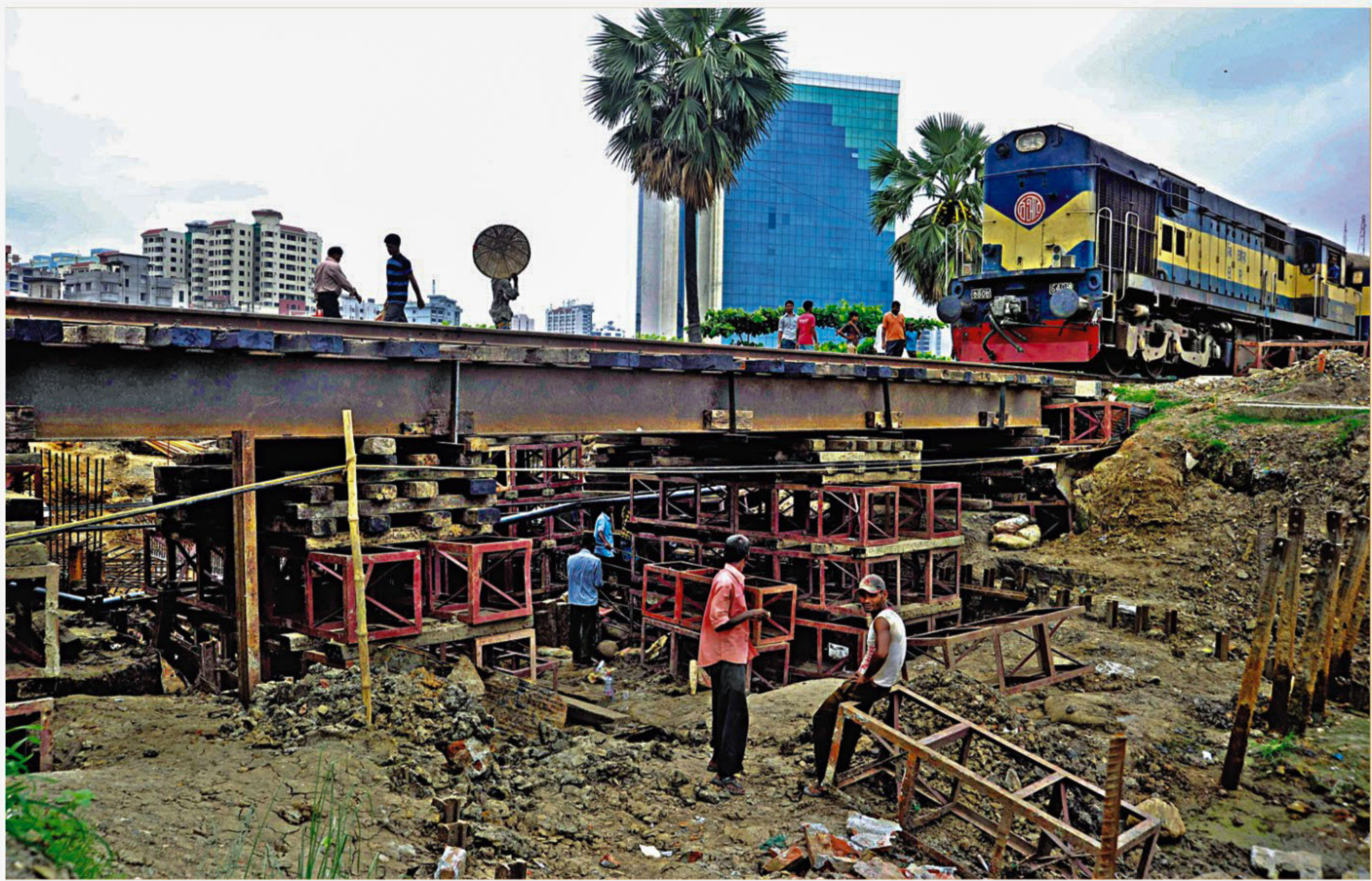
As a part of Hatirjheel water body reclamation project in the capital, an underground connecting channel is being built under the train tracks near FDC rail crossing to connect two sections of the water body. But trains still run on the tracks, during the construction underneath, risking accidents.
