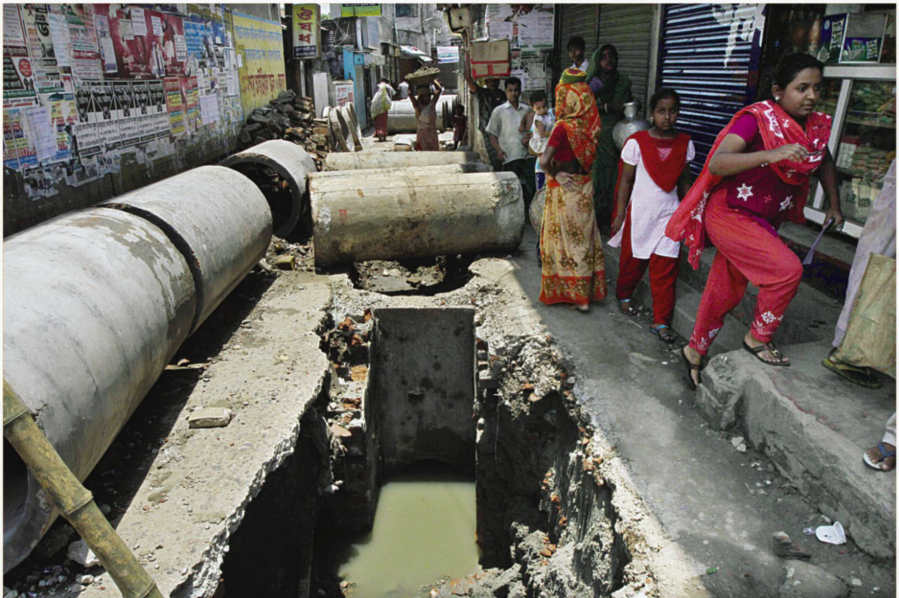
Local residents find it hard to pass this road at Golapbagh in the city dug up by Dhaka City Corporation to work on sewer pipes. The photo was taken yesterday.
