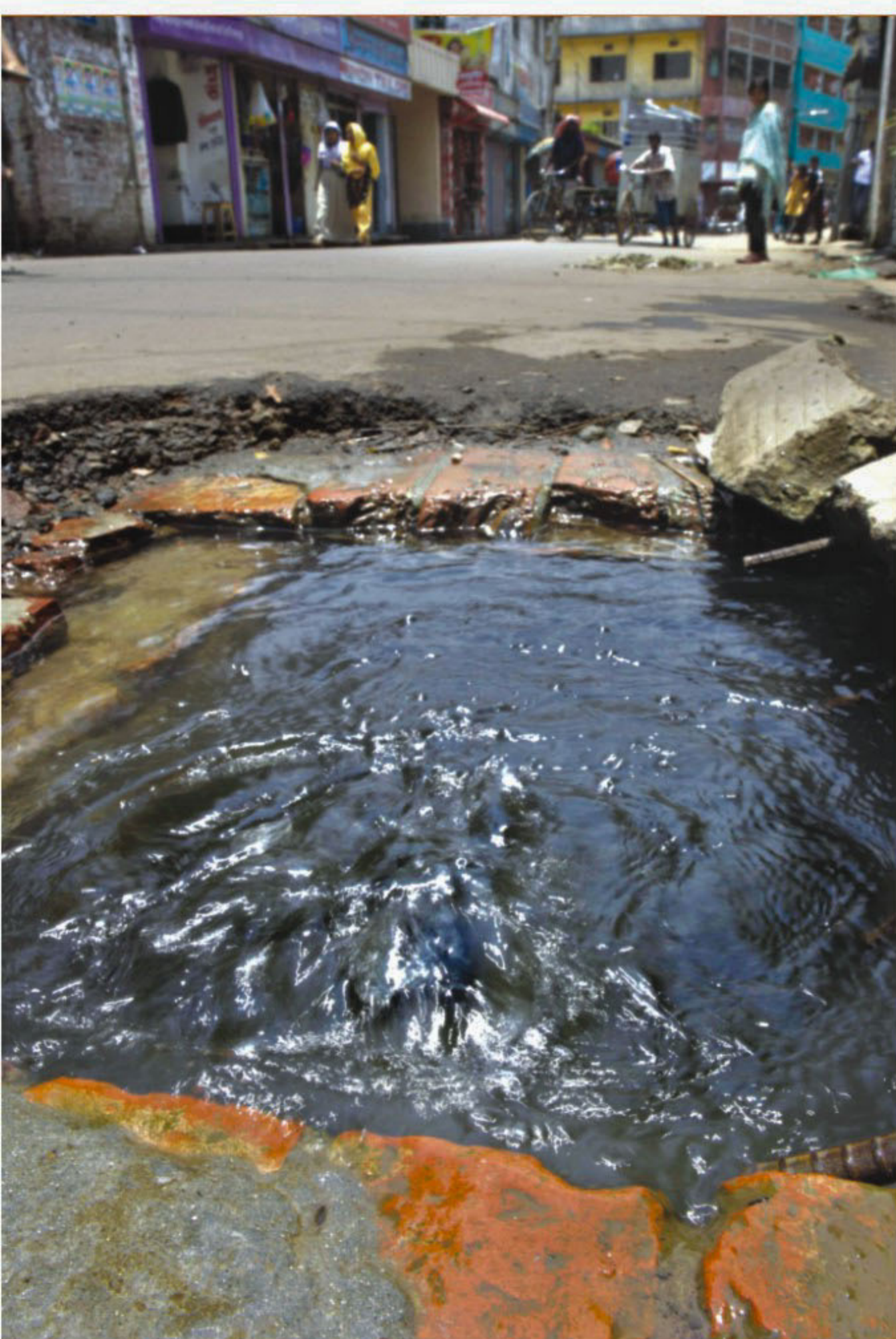
Supply water continues to leak from a broken Wasa pipe under Abul Hasnat road in Old Dhaka. The photo was taken yesterday.
