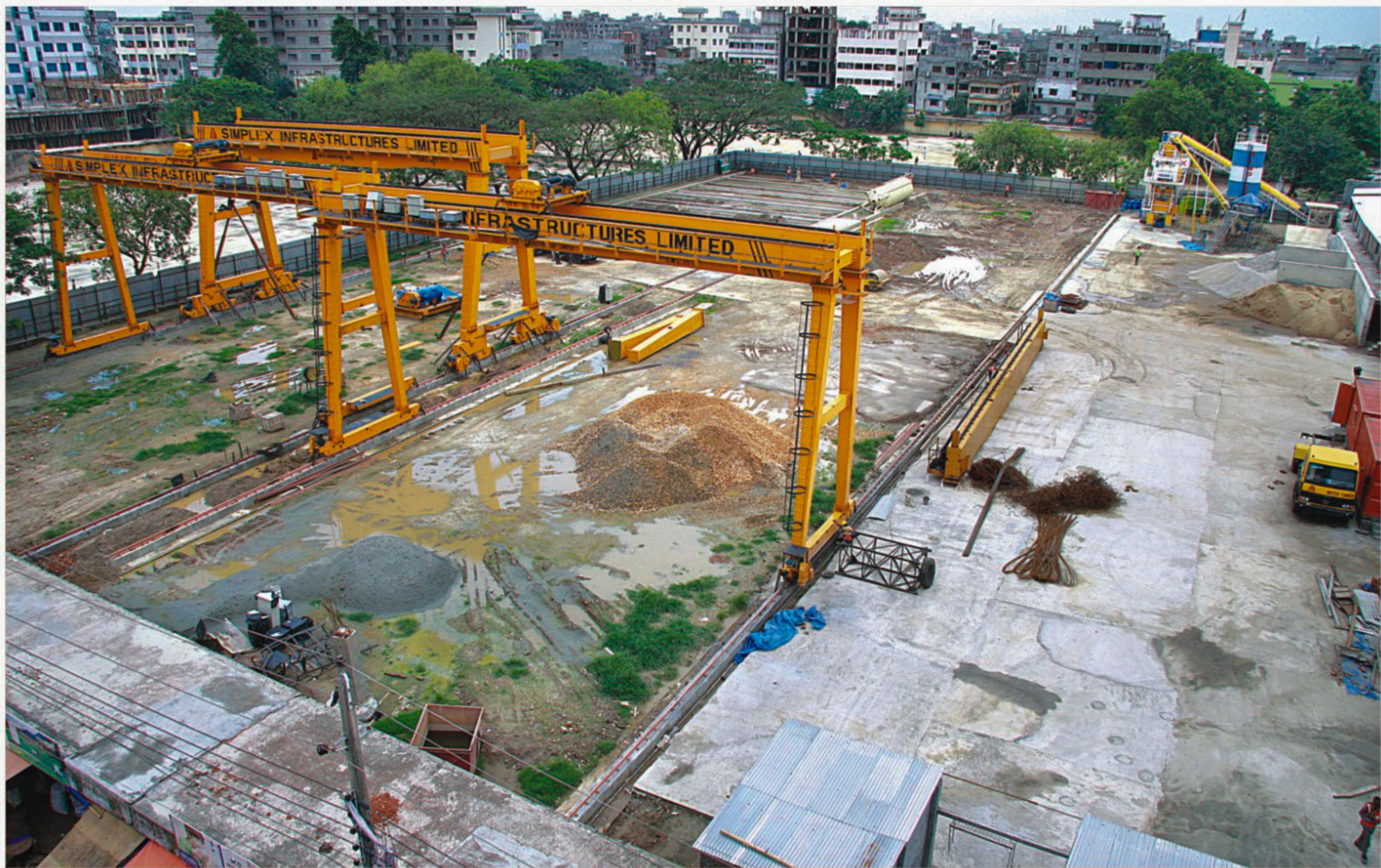
Construction materials of Jatrabari flyover piled up on Dhupkhola playground at Gendaria in the city. The photo was taken yesterday.
