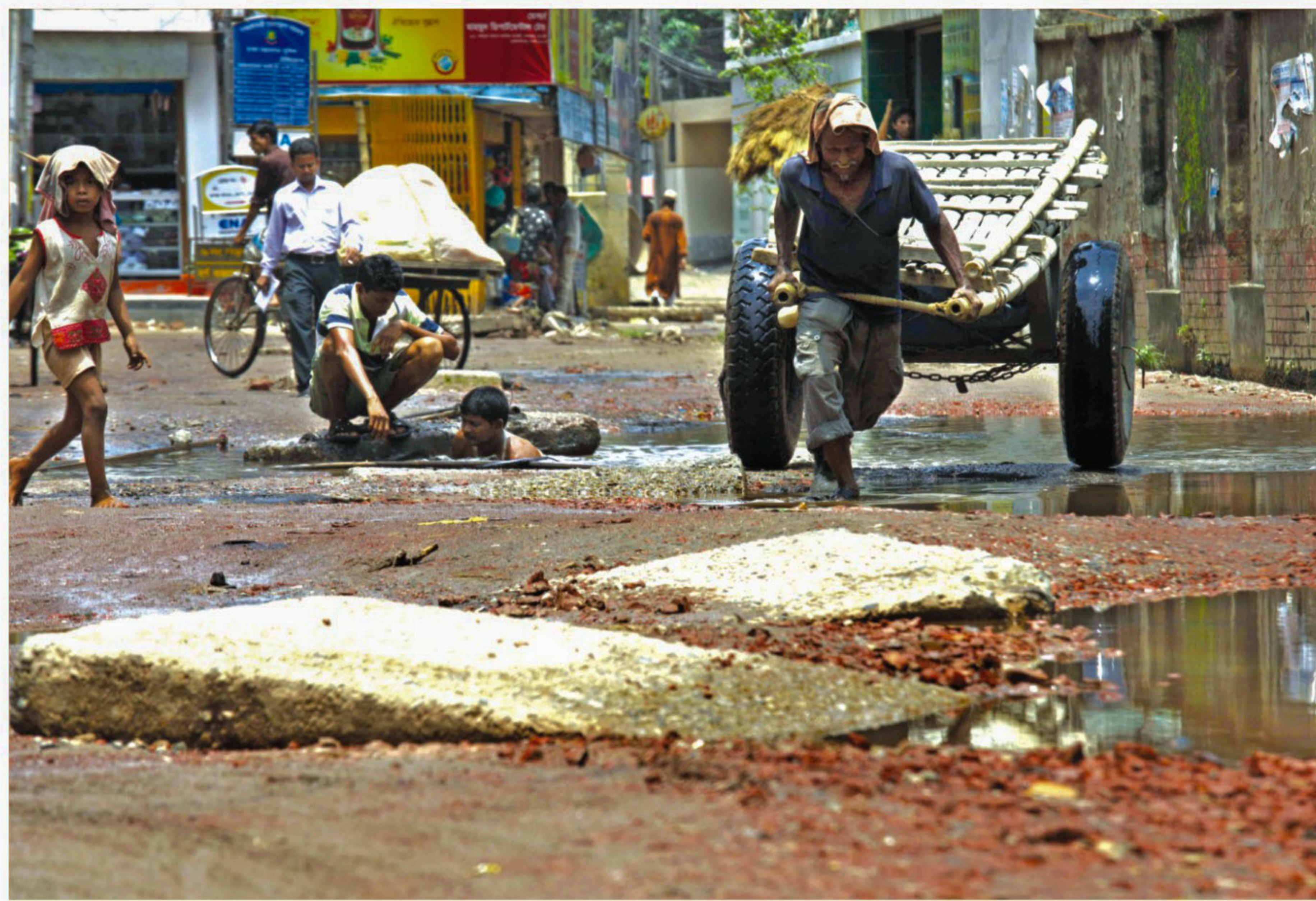
A man finds it hard to pull his cart on the pitted street with improperly positioned manhole covers in front of Bayetul Aman Housing Society in Adabor in the city yesterday.
