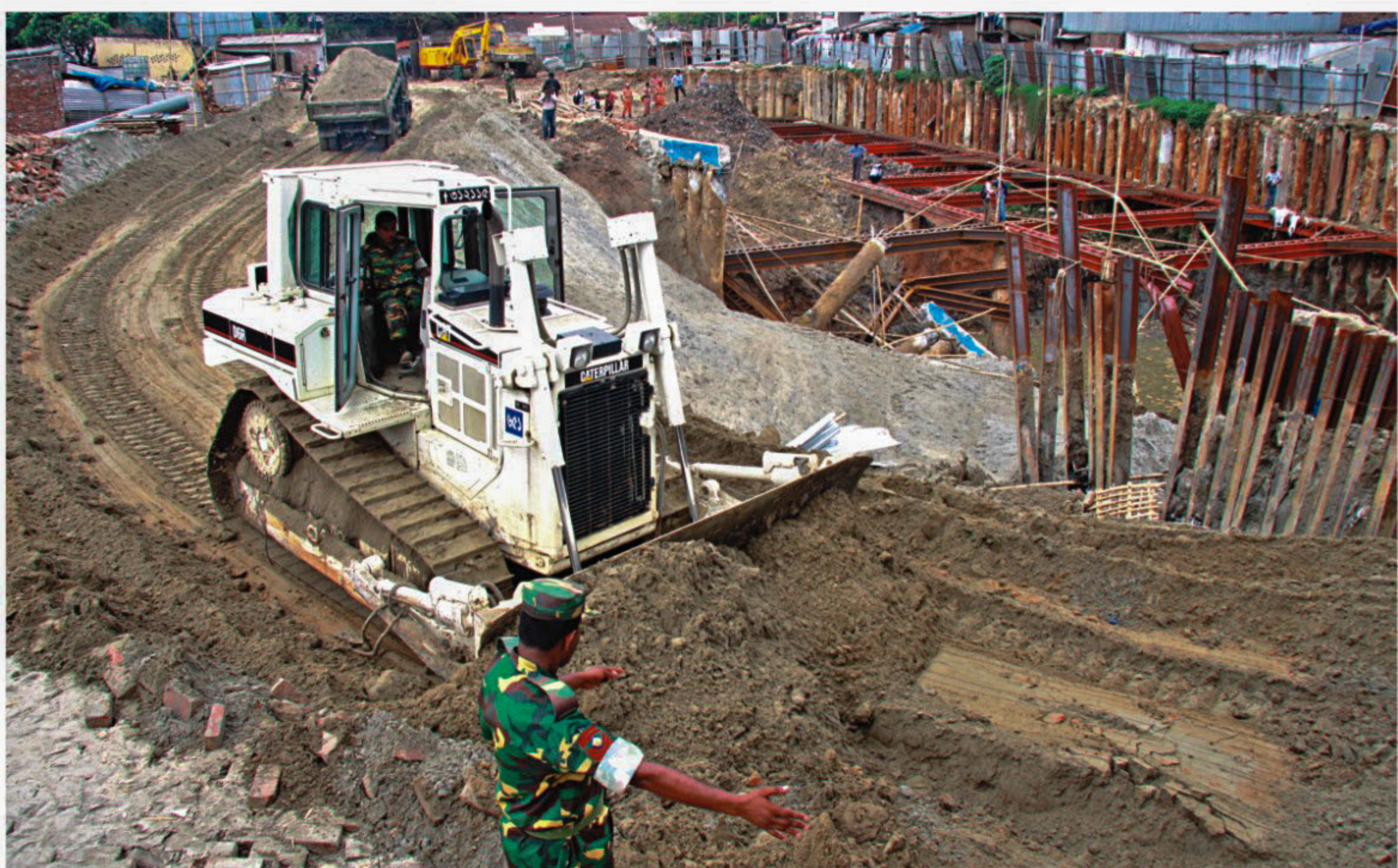
Army personnel filling up the gaping hole in the ground at Nakhhalpara in the capital where a large chunk of land subsided early Saturday putting several buildings at risk.
