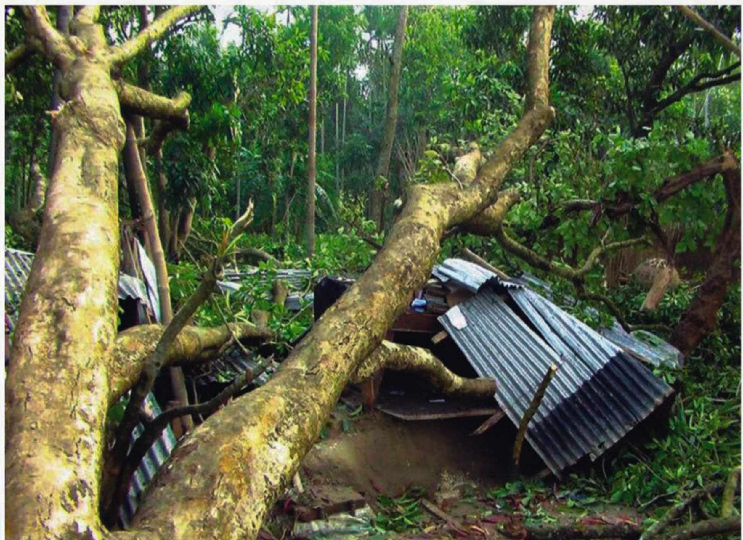
PHOTO: STAR A house was damaged as a big tree fell on it during Tuesday night's storm in Bera upazila of Pabna. The storm lashed five upazilas of the district.
