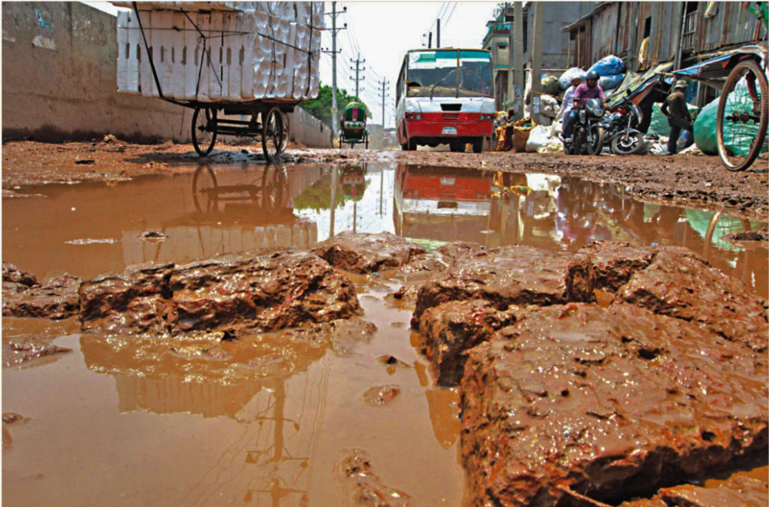
The dilapidated portion of Mitford-Gabtoi Beribadh road in Sowari Ghat area in the city is frequently waterlogged, causing immense suffering to the commuters. PHOTO: STAR
