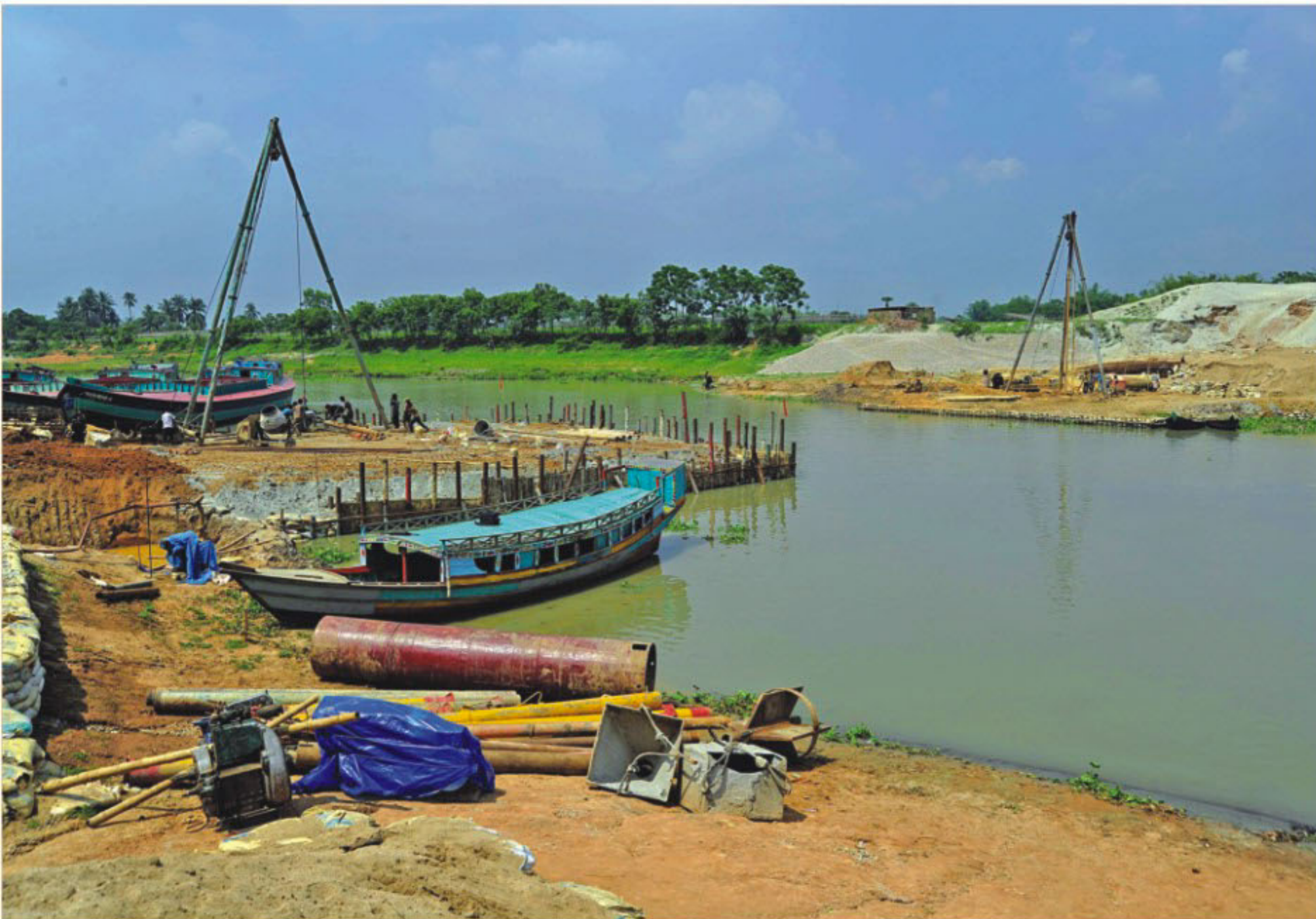
Almost two-thirds of the Balu river at Mashkul in Khilkhet has been filled up by Rajdhani Unnayan Kartripakkha to build a bridge. However, the Department of Environment has stopped the construction after The Daily Star ran a report on the issue yesterday.
