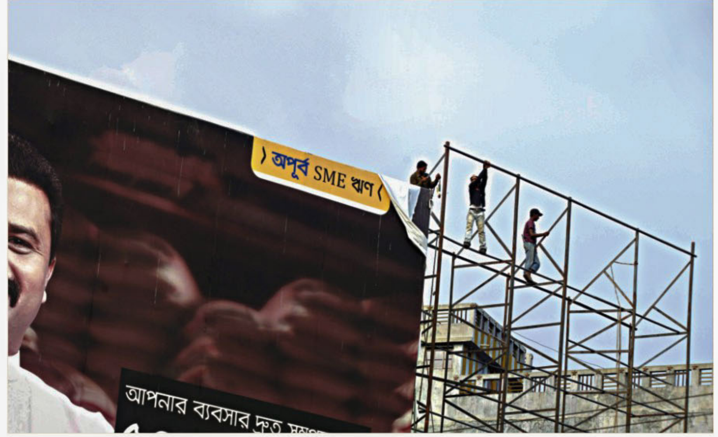
Workers setting up a hoarding on the roof of a building at Badamtoli in the capital yesterday without safety gear. Such unsafe construction work often leads to fatal accidents. Three workers died Tuesday after falling from an under-construction building in the city's Bashundhara area. PHOTO: RASHED SHUMON
