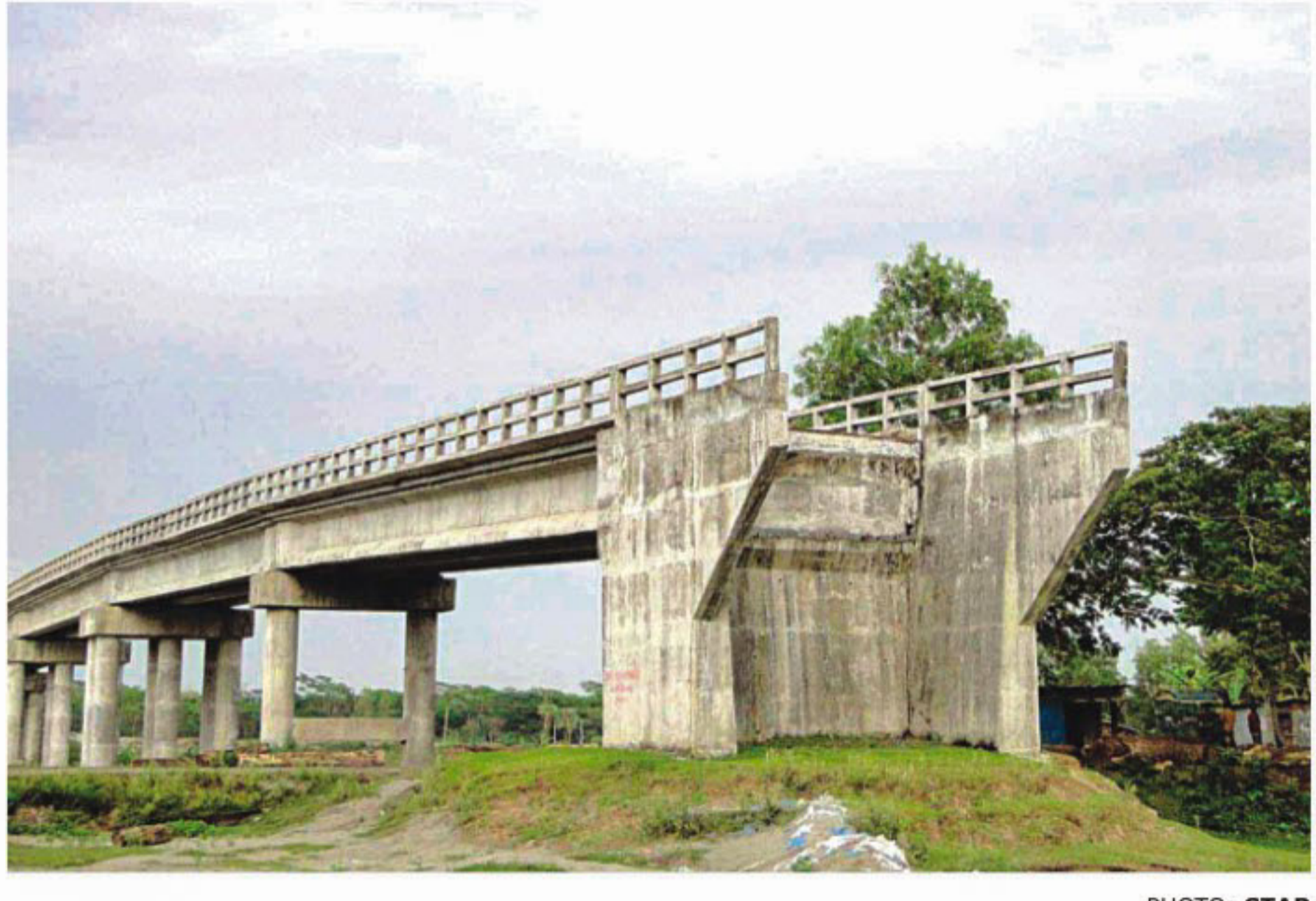
PHOTO: STAR This impressive bridge over Nurainpur River in Baufal upazila under Patuakhali district remains without any utility to the locals as no approach road has been made three years after its construction.
