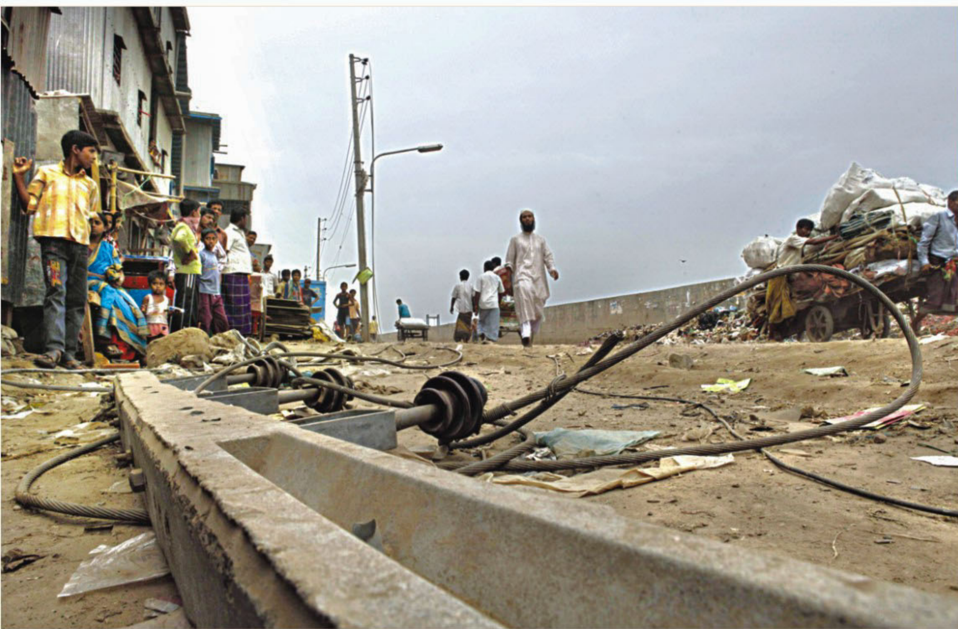
This electric pole on Islambagh Beribadh road of Lalbagh area in the city was rammed down by a truck on Sunday evening, injuring two people and severing power connection to the area. Power was still to be restored till 4:00pm yesterday when this photo was taken.
