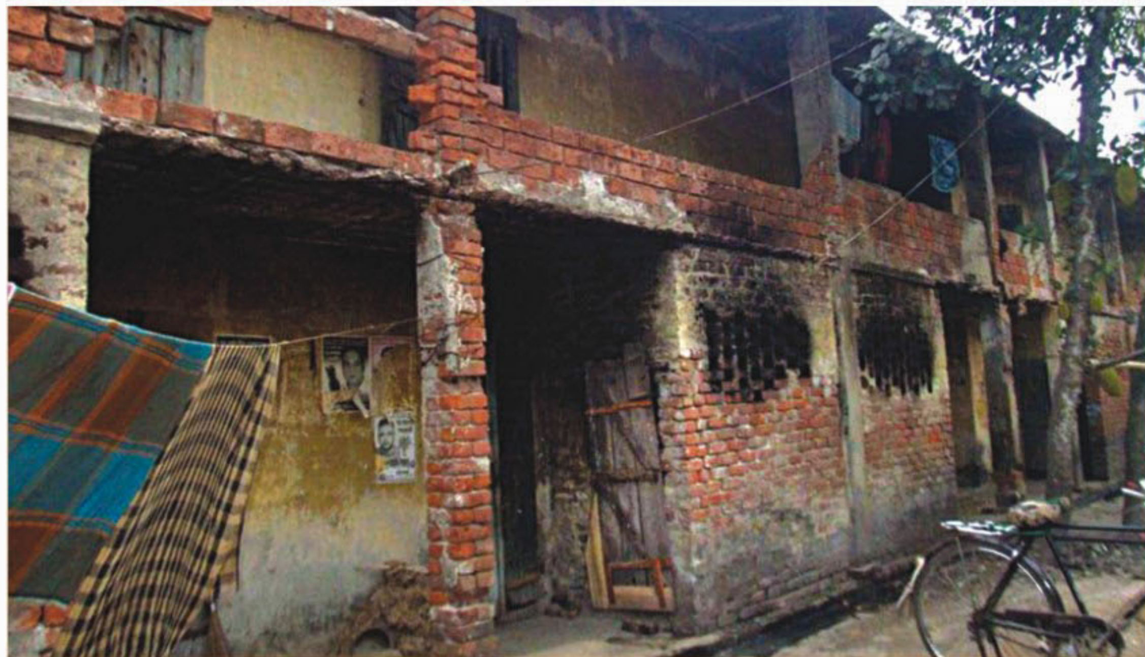
STAR Workers and employees of Platinum Jubilee Jute Mill in Khulna live in such dilapidated buildings. The authority is unable to renovate five such buildings due to a fund crisis.
