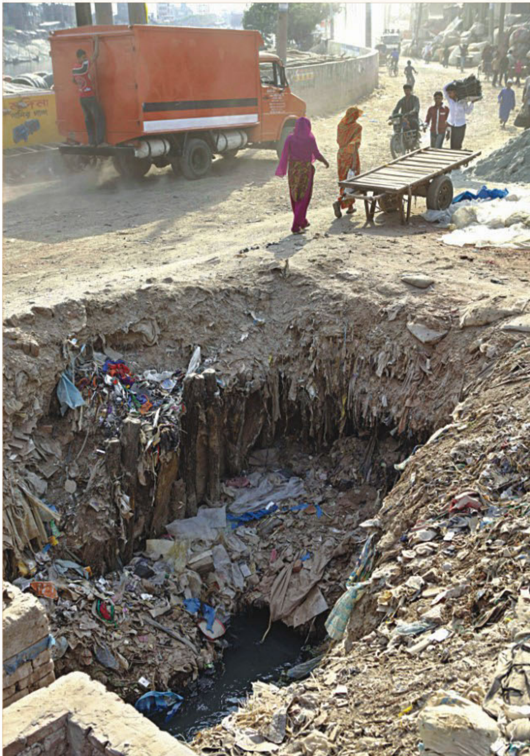
This gaping hole on Beribadh Road, which is in a sorry state from Abu Bazar to Aminbazar, at Islambagh in the city poses a hindrance to commuters and a threat to vehicles. The photo was taken yesterday.
