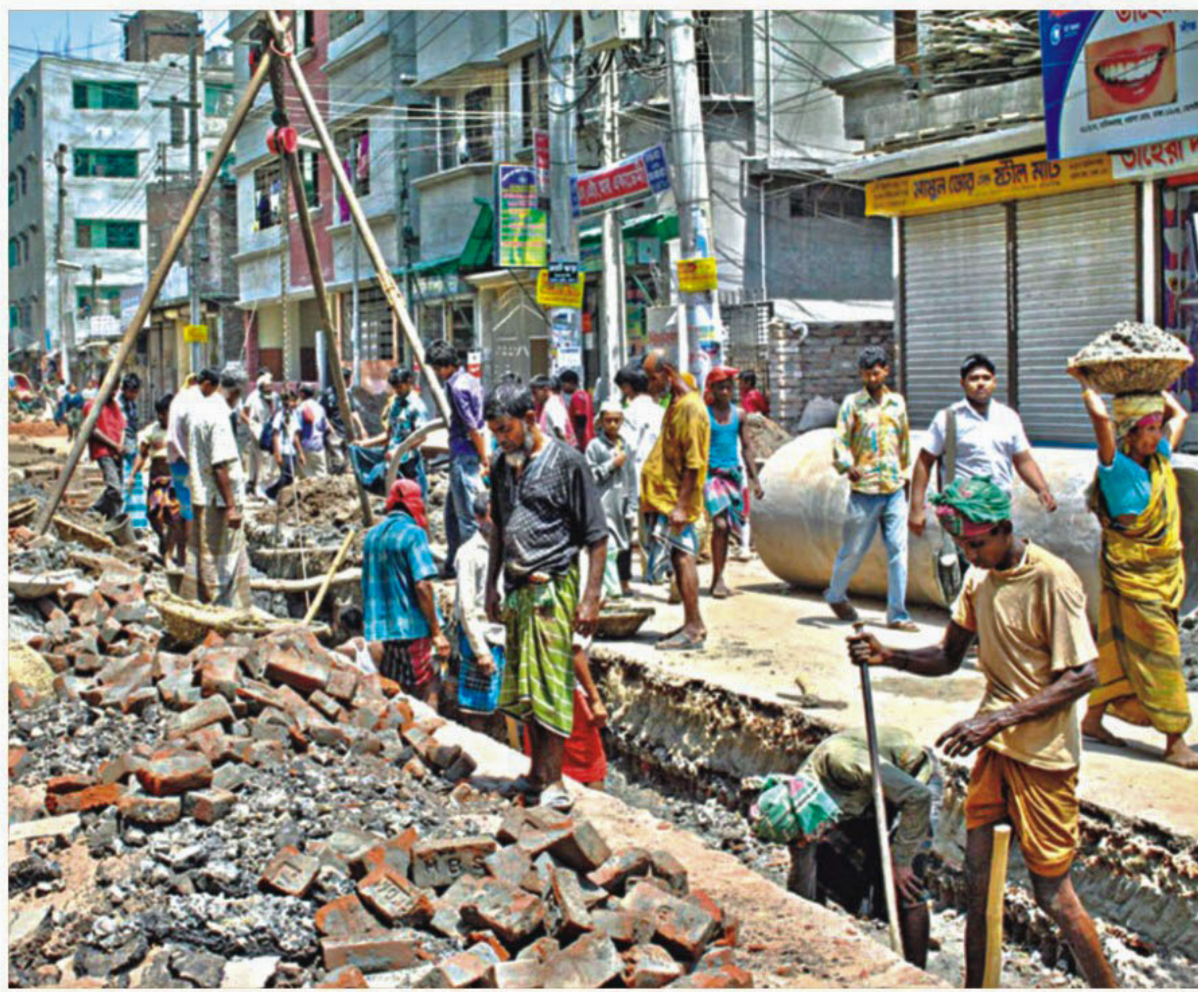
Sewerage works in progress in the city ahead of the monsoon. The photo was taken at Maniknagar yesterday.
