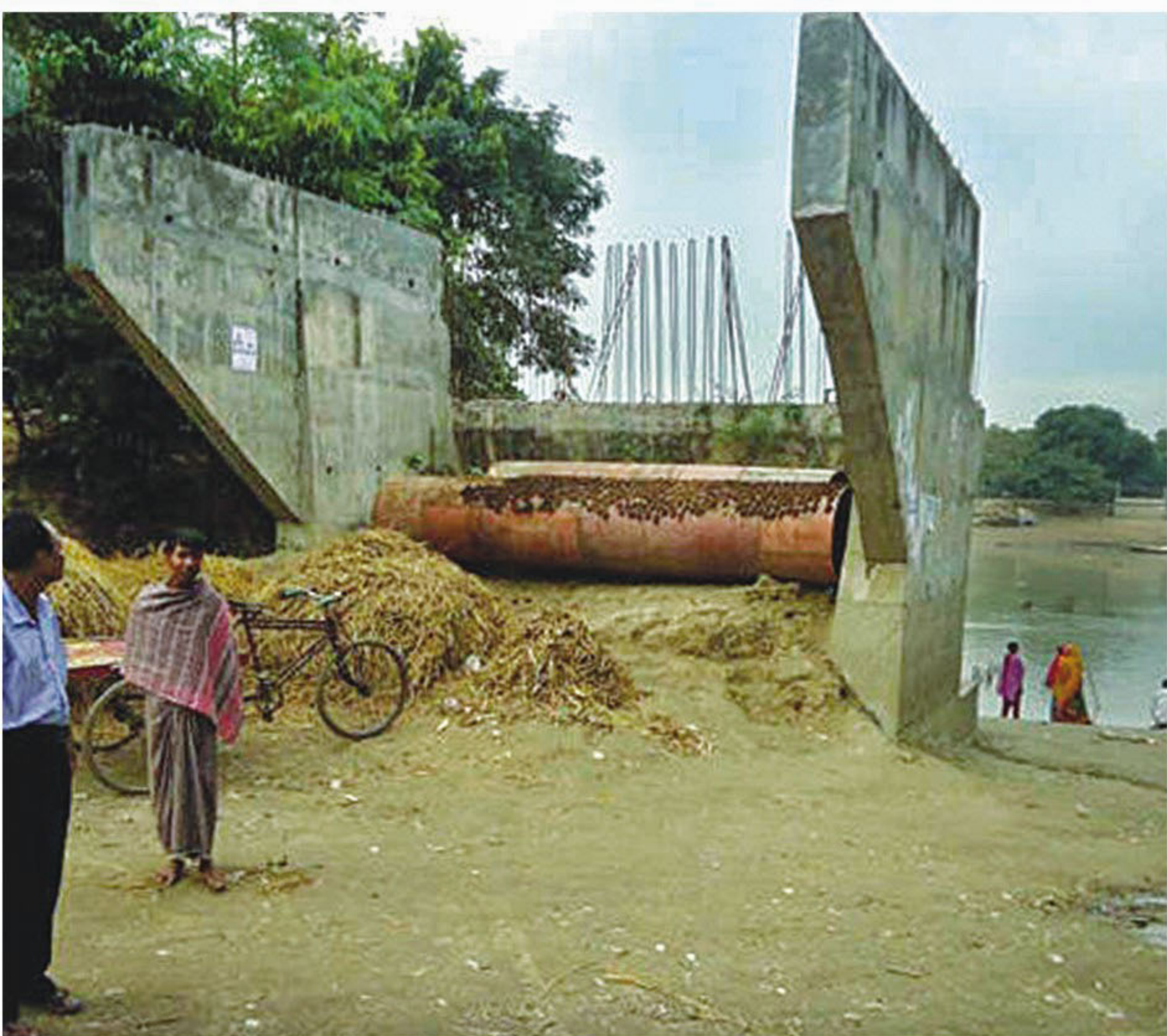
Left incomplete after construction of a few pillars two years ago, this bridge over Boral River at Gunaigachha village in Faridpur upazila of Pabna district remains a mockery to a large number of people in four unions of surrounding areas.
