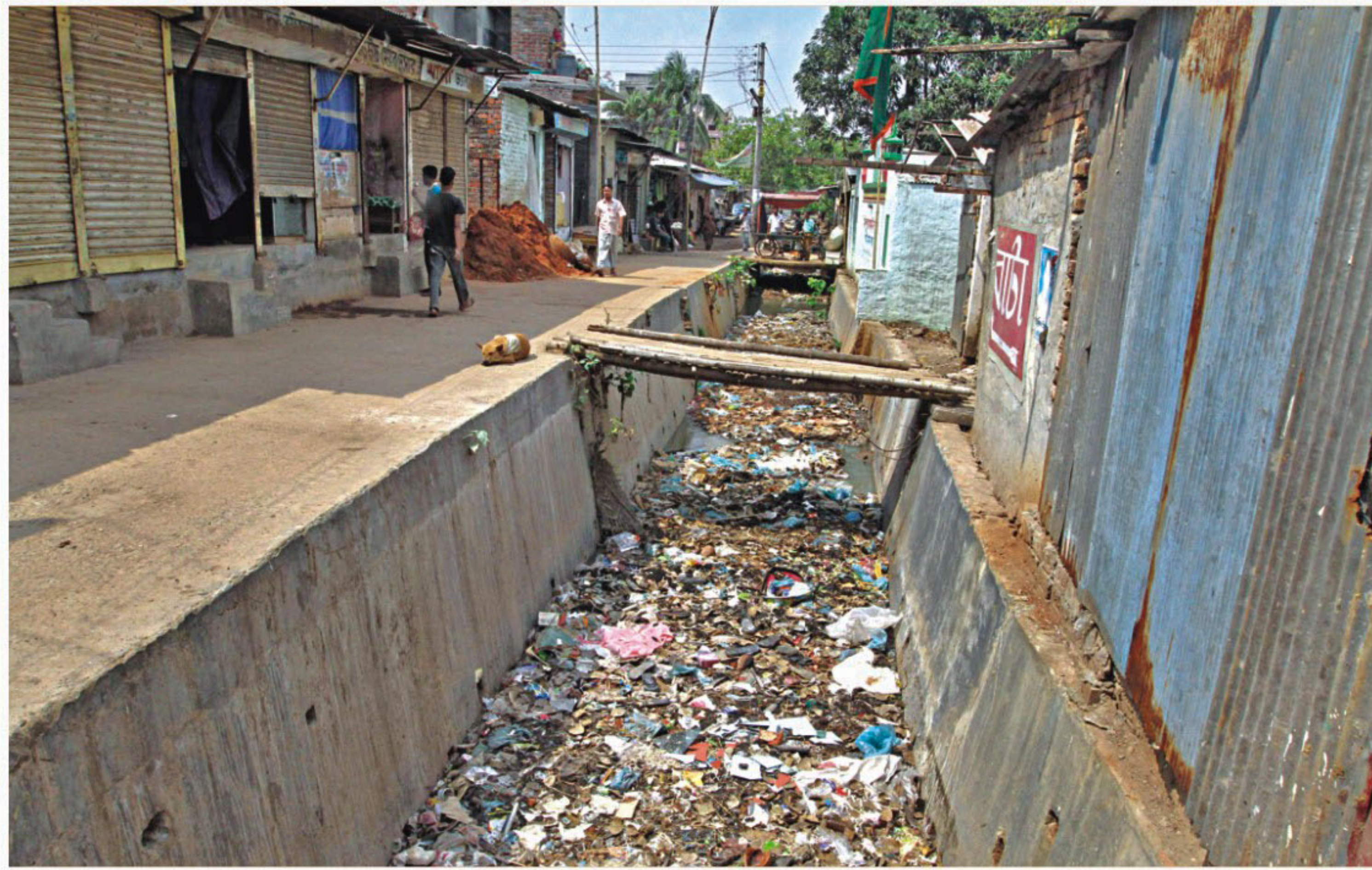
This open drain of Dhaka City Corporation in Muslim Bagh area of Mirpur 12 in the city is full of garbage, releasing stench over the area. Locals claim that this drain sometimes overflows filling adjacent roads with the waste.
