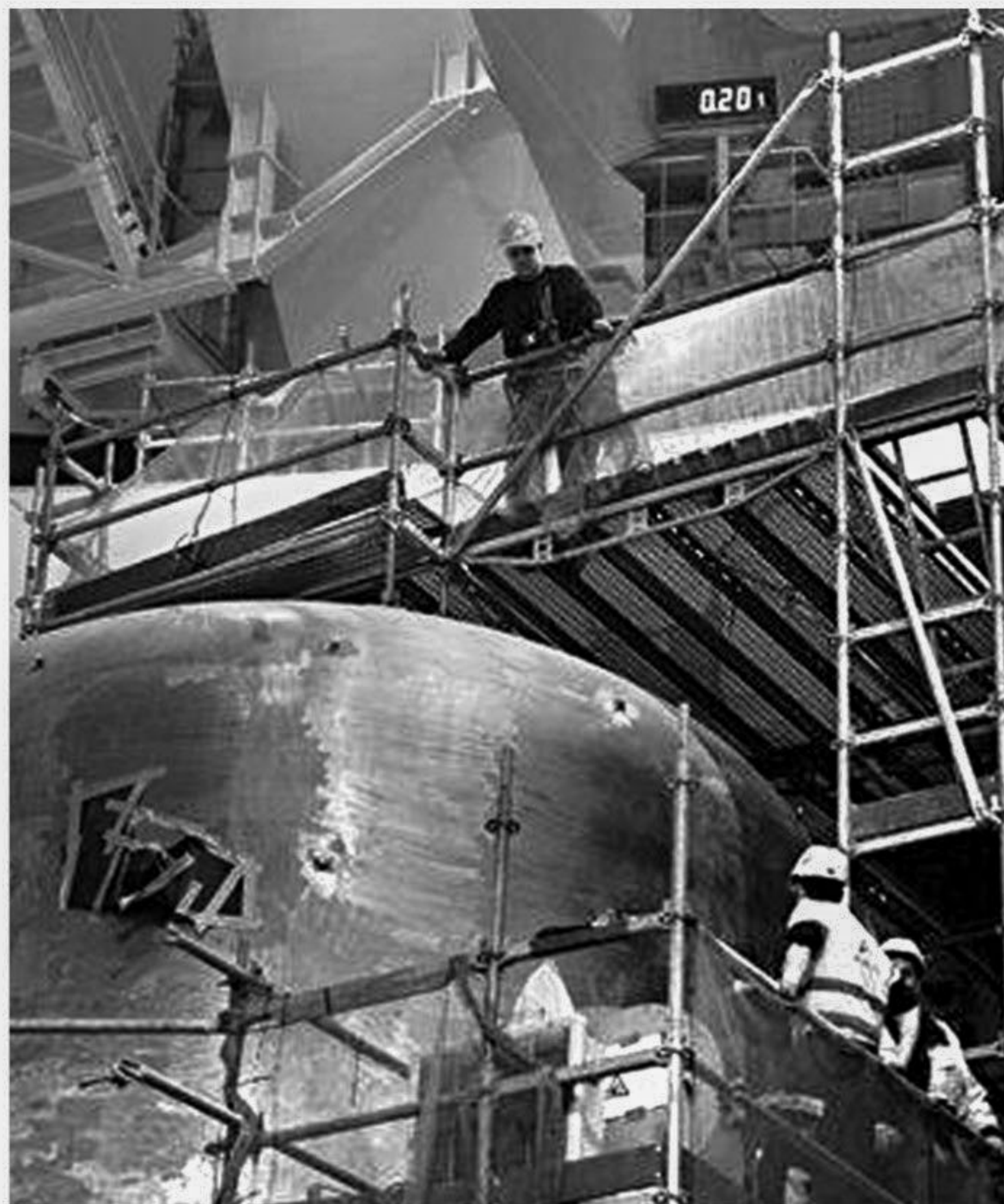
Contractors work in the reactor building at the construction site of the nuclear power plant Olkiluoto 3 'OL3' in Eurajoki, south-western Finland on March 23.
