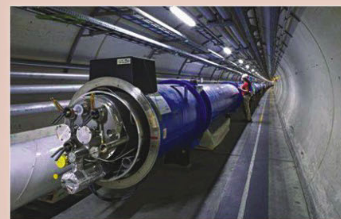
A worker inside the LHC tunnel working on the large magnets that guide particles around the LHC loop
