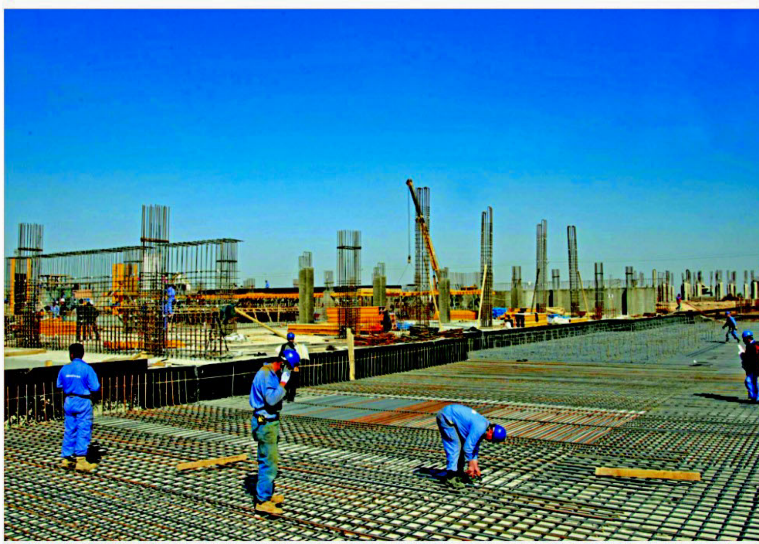
Iraqi construction workers build the new Culture Palace in the central Iraqi holy city of Najaf.
