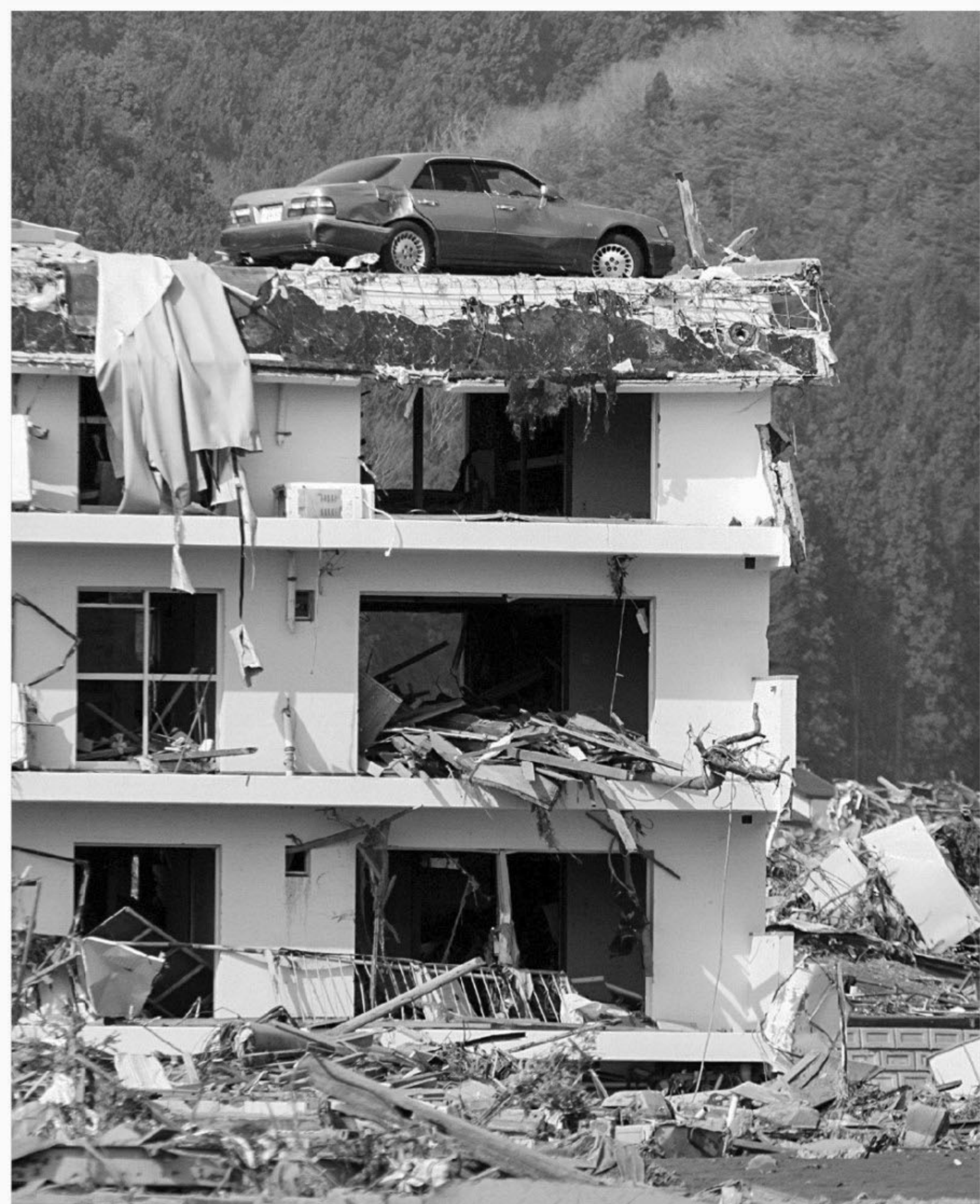
A vehicle sits on a three-story building at Tsunami-hit Minamisanriku town of Miyagi prefecture after yesterday.
