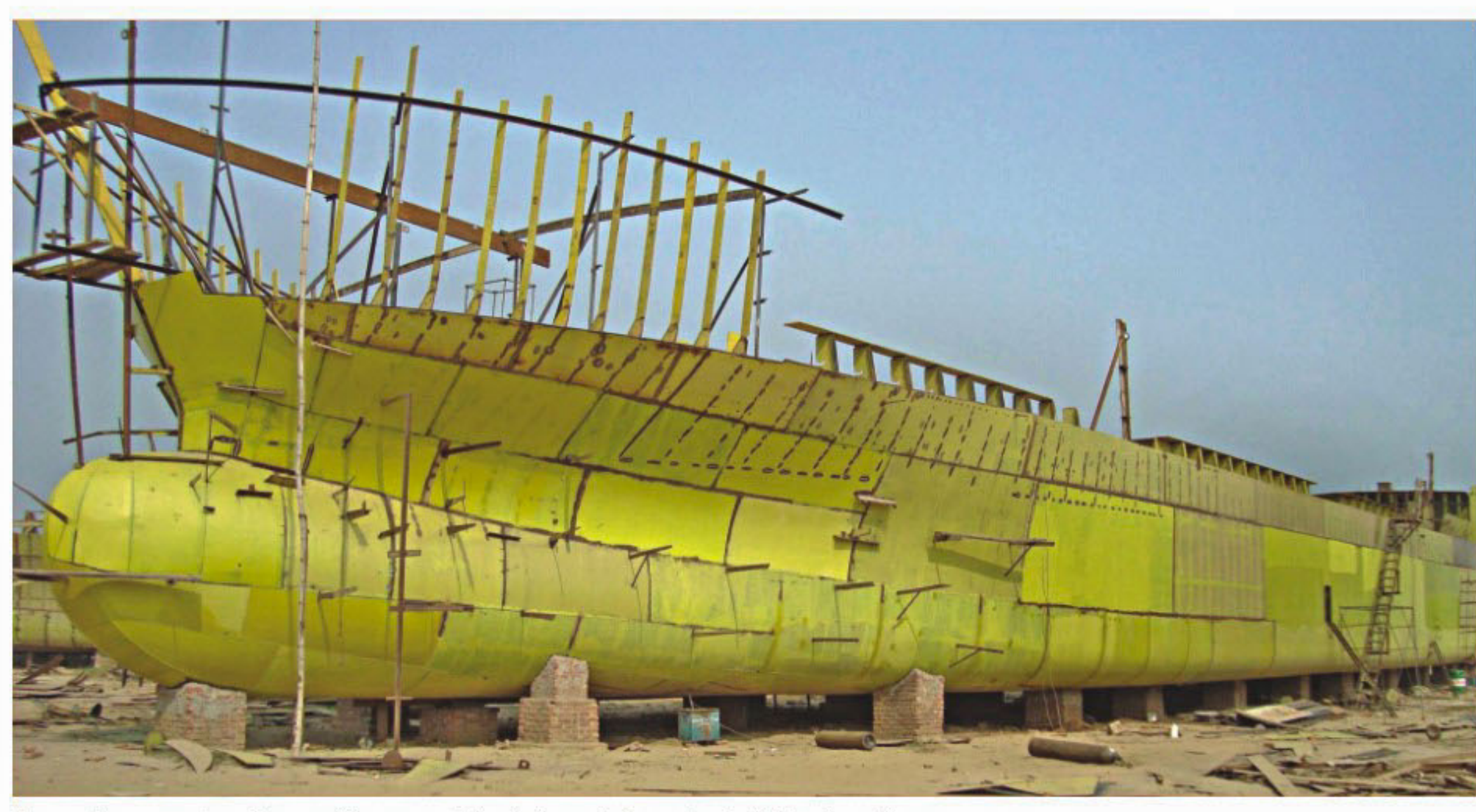
An under-construction water vessel is pictured at a plant of Meghna Group.
