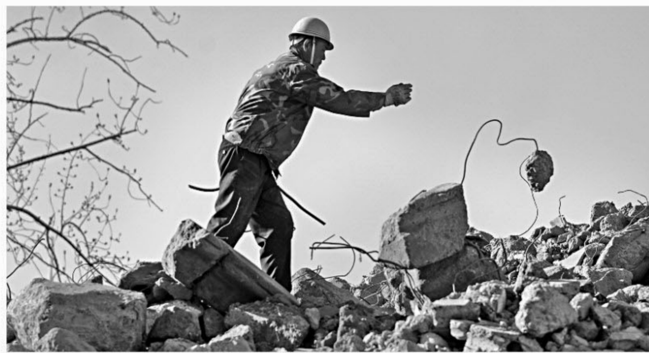
Workers demolish an old house at a construction site in Beijing yesterday. China will invest around $200 billion this year in affordable housing, a senior official said, as Beijing struggles to address mounting public concern over runaway property prices.
