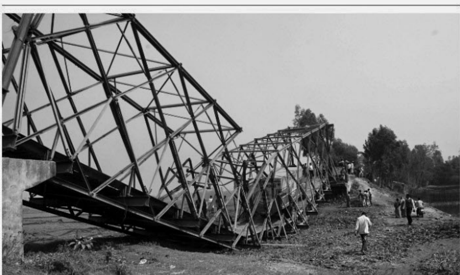
A bailey bridge on Bogra-Gabtolli Road collapses due to heavy pressure of a cement-laden truck in Kholisagura area under Gabtoli upazila of Bogra district yesterday morning.
