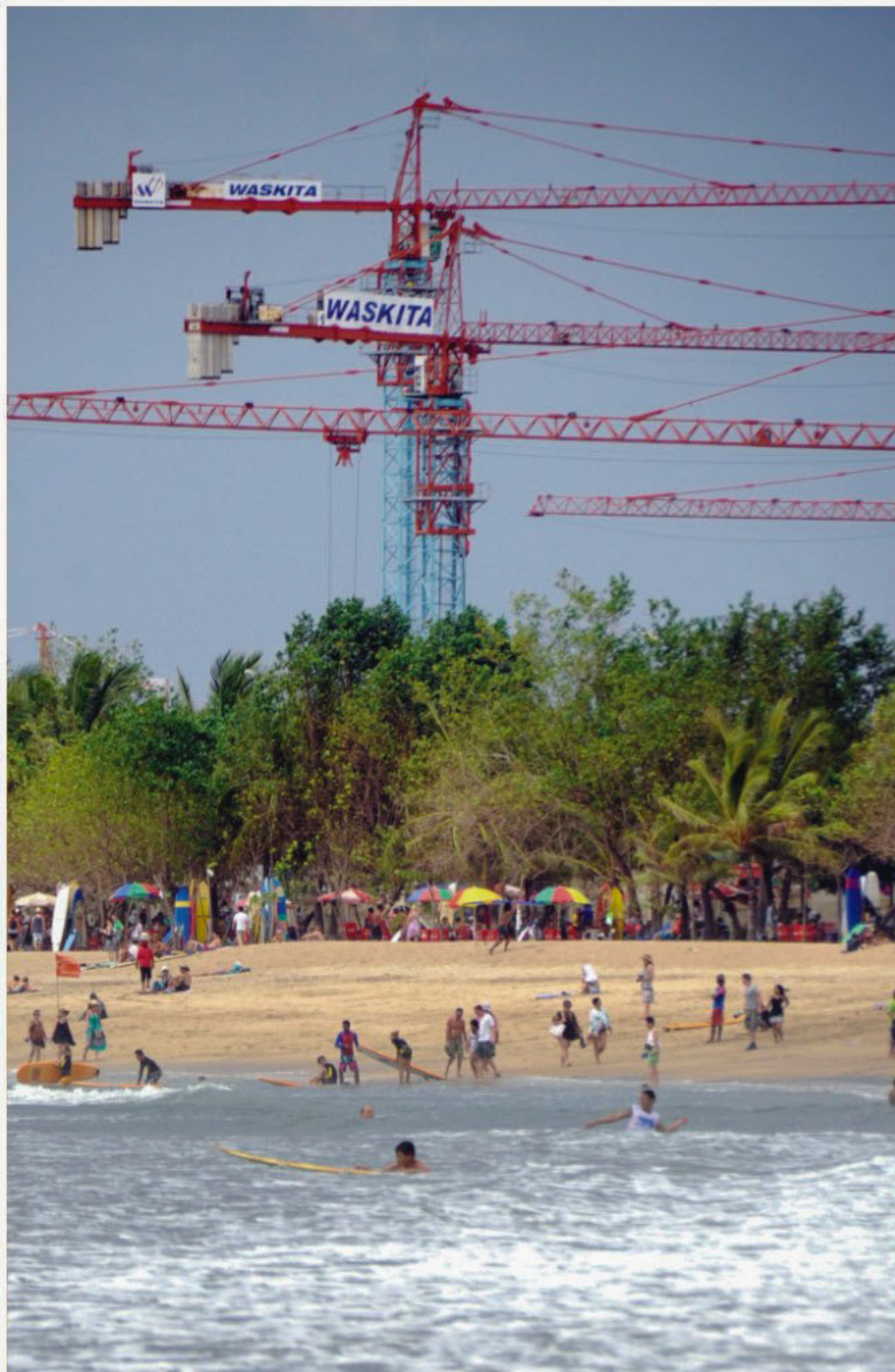
AFP Tourists flock to Kuta Beach on the resort island of Bali while in the background construction cranes are busy at work on the massive beachfront development dubbed the Beach Walk.
