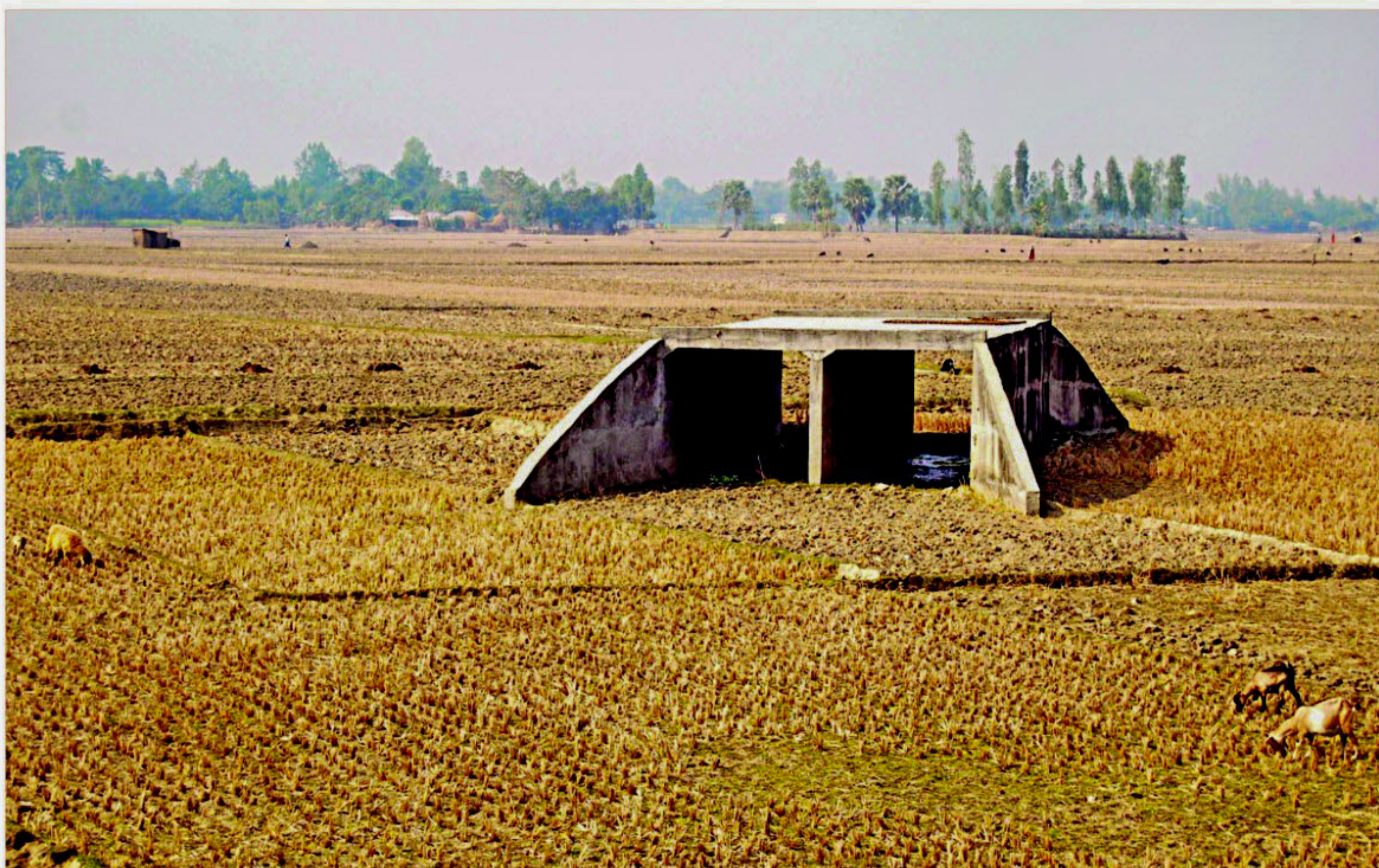
During the tenure of the last BNP-Jamaat government, this culvert was built at a place with no road. The photo was taken at Balia Dighee of Gabtoli upazila in Bogra. Bridges and culverts like this one were built all over the upazila.
