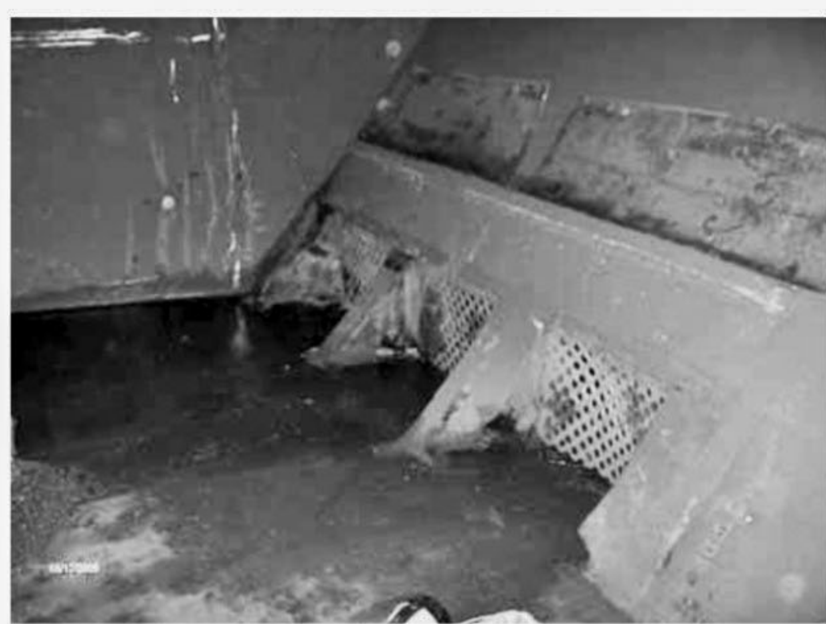
Bilge well with highly polluted bilge water.
