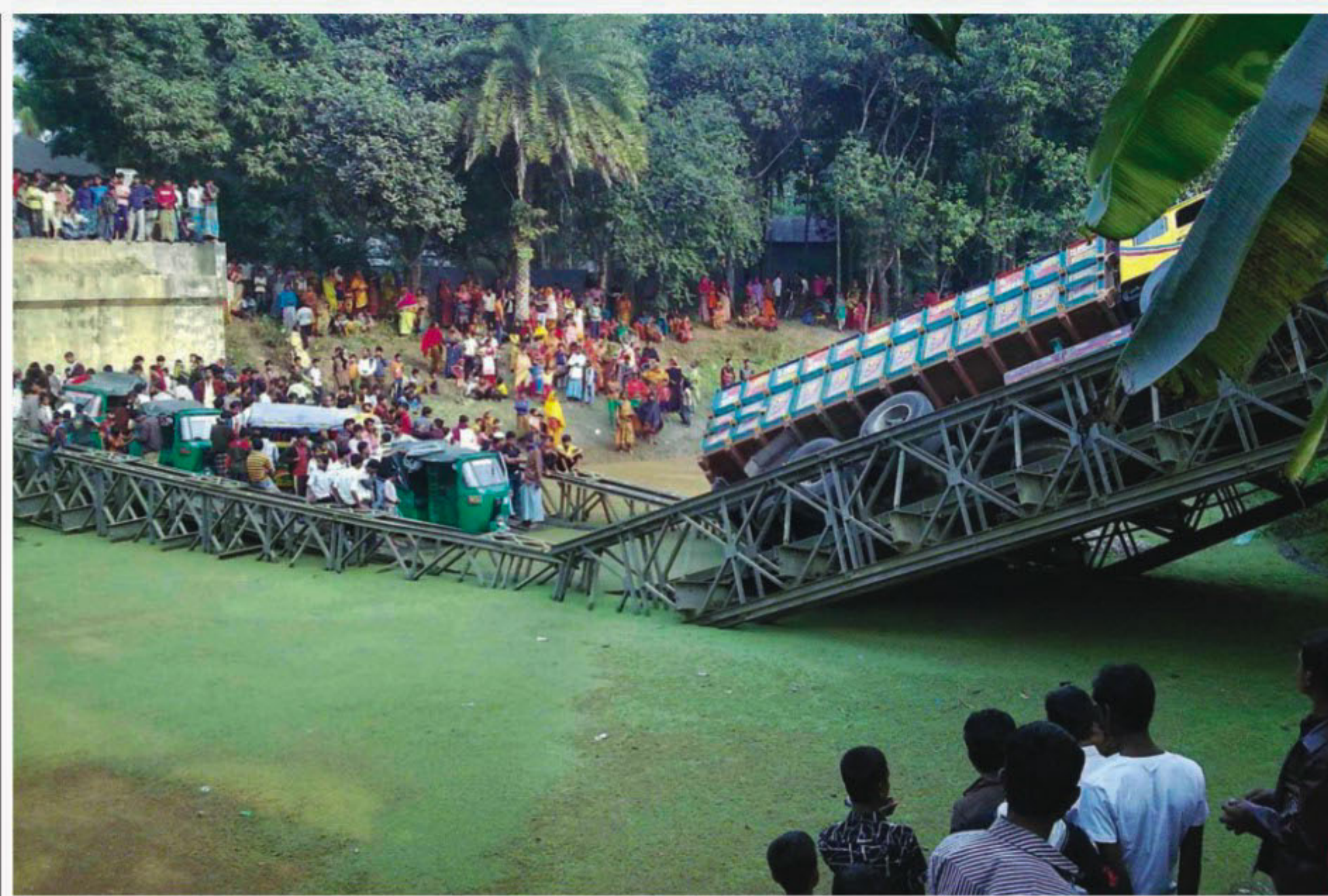
PHOTO: STAR The bailey bridge near Elasin Bazar in Delduar upazila of Tangail district collapsed under the pressure of a stone-laden truck on Sunday afternoon, causing death to one and injuries to 15 others. Vehicular movement on busy Tangail-Aricha road has remained suspended following the accident.
