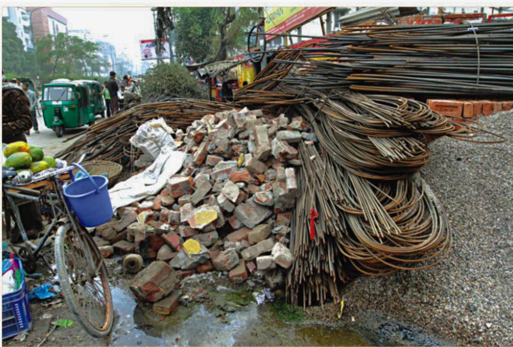
Pedestrians suffer as the construction materials are heaped all the way on the footpath of Road No 9 in the city's Dhanmondi. The photo was taken yesterday.
