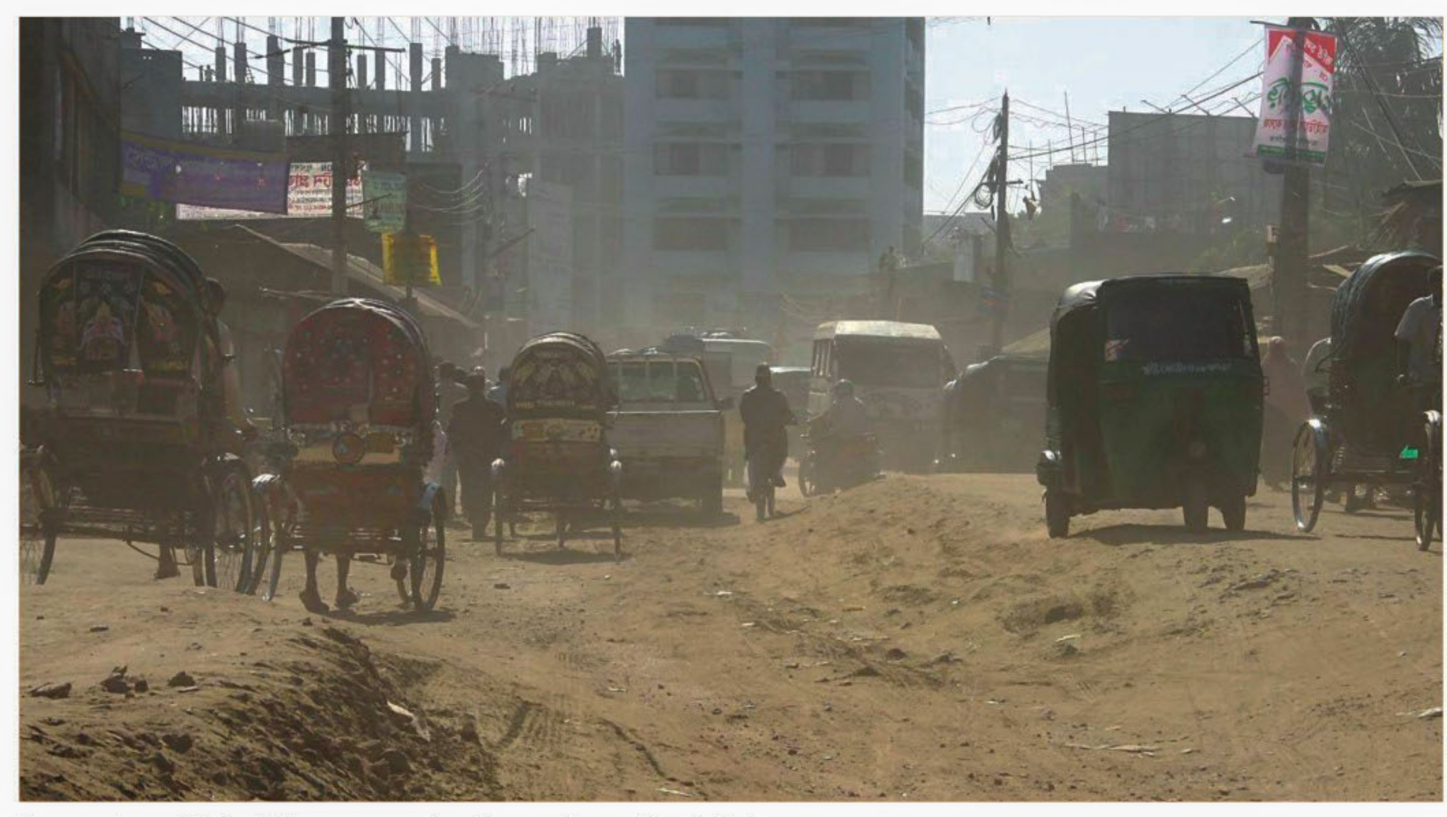
Kapasgola road in bad shape as construction work remains stalled.
