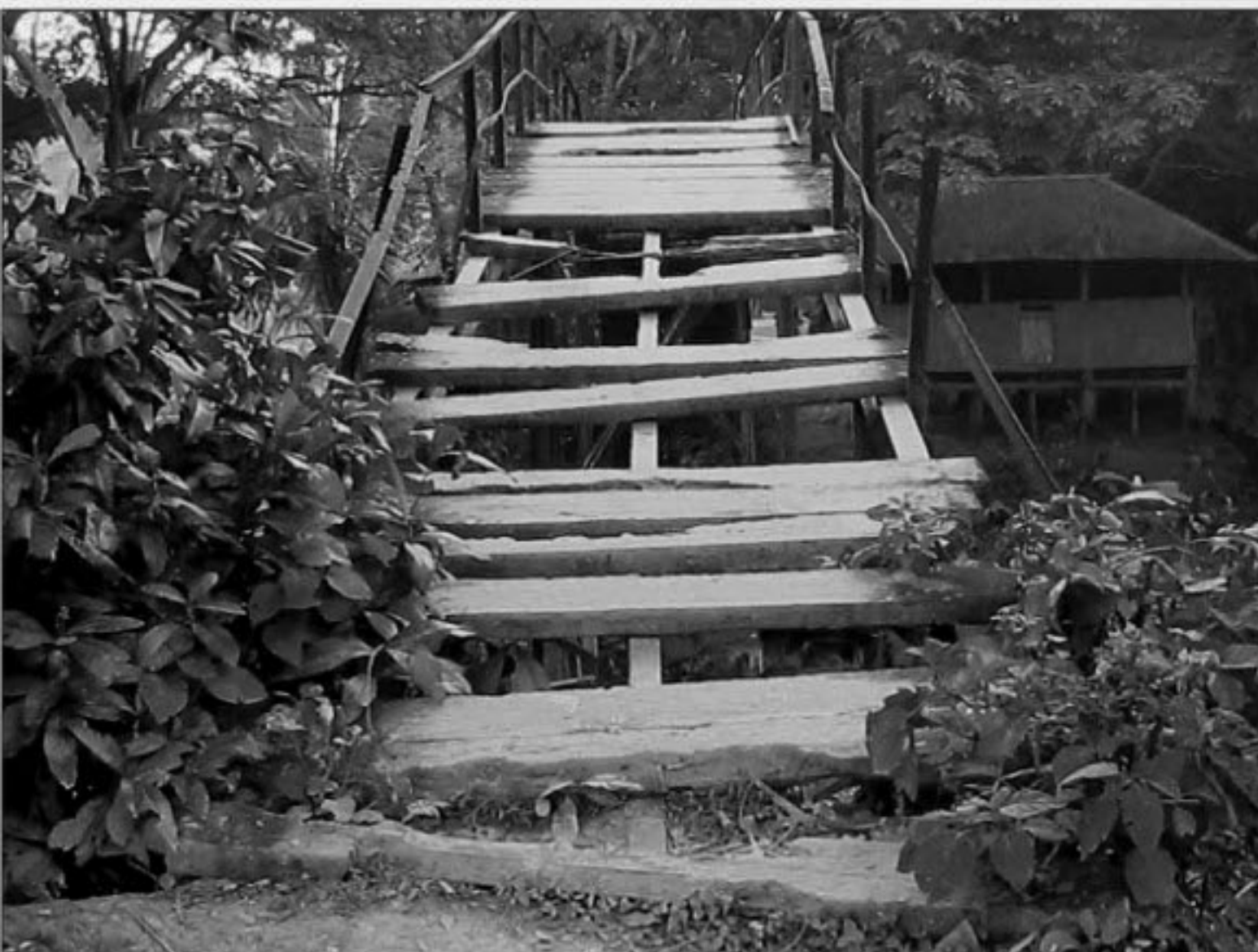
The bailey bridge across Kewabunia canal on Dashmina-Nehalganj road in Patuakhali district has remained in a awfully dilapidated condition while the bridge across Daspara canal on the same road lacks approach road, posing serious risk for the users.
