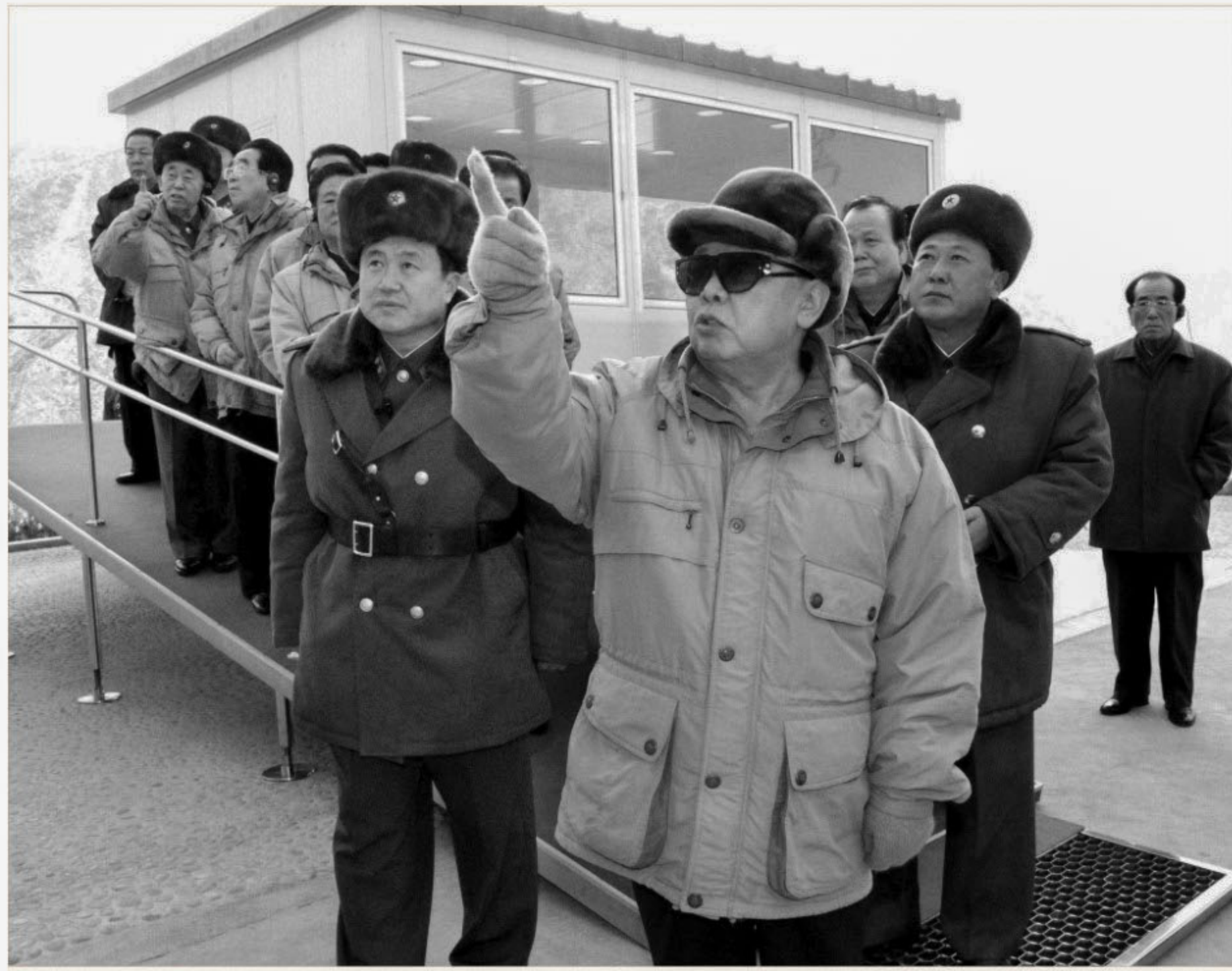
This undated picture released by North Korea's Central News Agency on December 22 and distributed by Tokyo's Korean News Service yesterday shows North Korean leader Kim Jong-il (C) visiting a construction site of the Huichon power station in Chagang Province. North Korea has declared a public holiday to mark the birthday of leader Kim Jong-il's youngest son, a report said yesterday, as the regime grooms him to take over power from his father.
